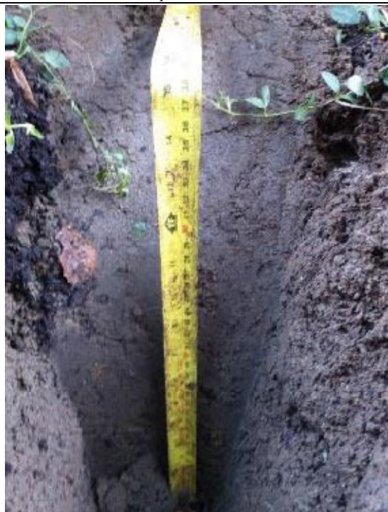
Photo 7: Verification Point 108, showing the greater depths of cover in the courtyard areas of soft landscaping with the plant beds.
