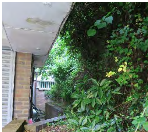
Gap between Brunner House and Boundary Wall
