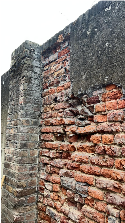
Fig 2: Photo of the internal face of the wall with render removed
