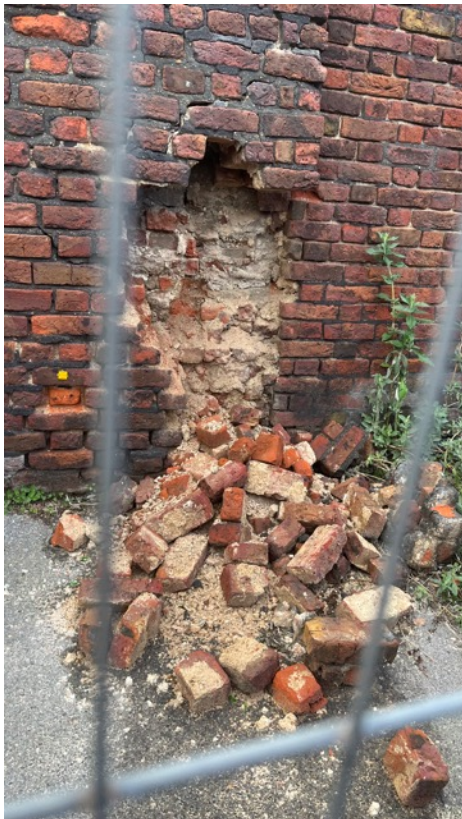
Fig 1: Photo of the wall collapsing
