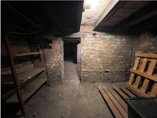
Fig.4 : Existing cellar to front of property - low headroom
