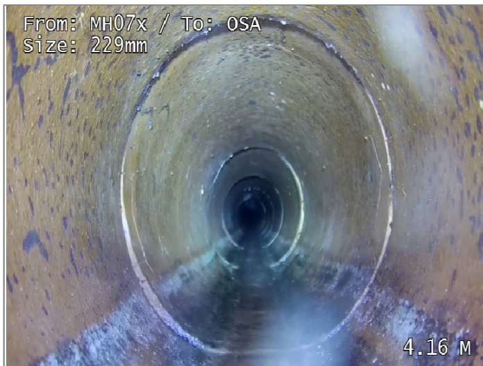
Joint displaced medium
