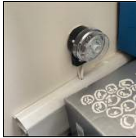
Figure 15 – Time clock located within office area
