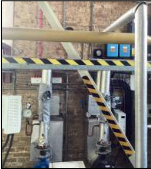
Figure 18 – Time clock controls located behind low level steel frame with hazard tape
