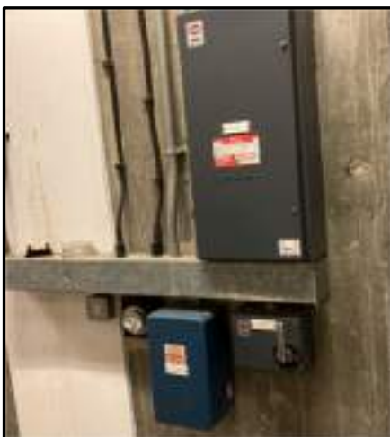
Figure 16 – D.F.B 1X4 time clock controls
