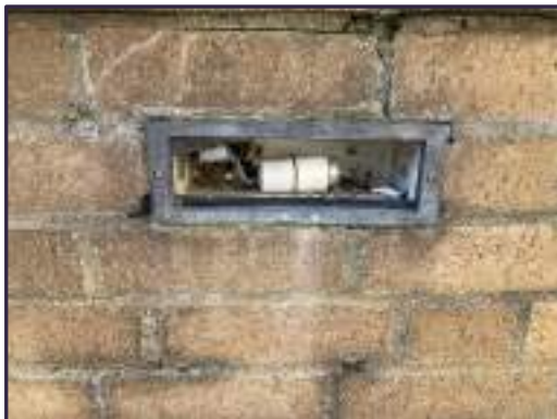
Figure 31 – Damaged external lighting located with blockwork wall
