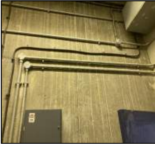
Figure 22 – Overhead services located in ground floor plantroom
