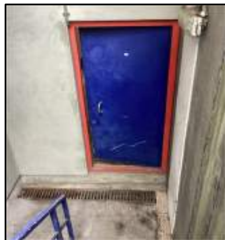
Figure 17 – Corridor access door to D.F.B 1X4 time clock controls
