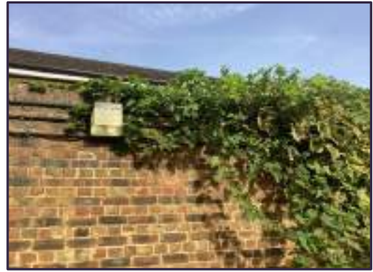
Figure 26 – External lighting cabling surrounded by foliage
