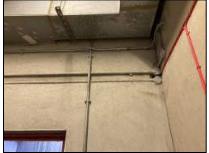
Figure 23 – Overhead services located in basement lobby corridor with time clock cabling behind ducting
