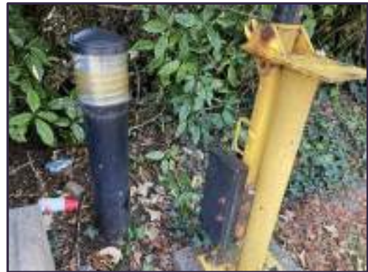
Figure 32 – External lighting located by security barrier and rubbish present
