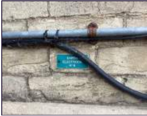
Figure 25 – Earthing electrode adjacent to lighting cabling
