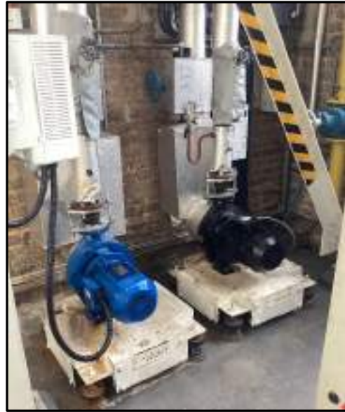
Figure 19 – L.T.H.W pumps located in ground floor plantroom
