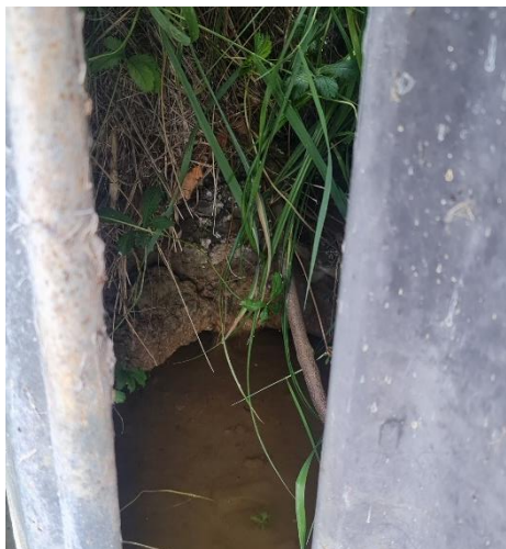
Plate 2: Gap within canal piling at western end of site.
