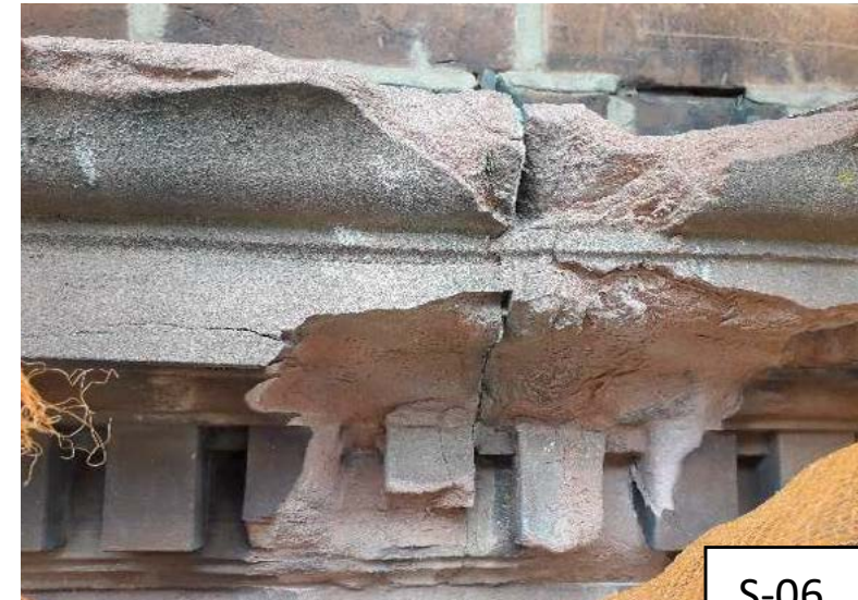
risk of falling masonry - facade repairs necessary
