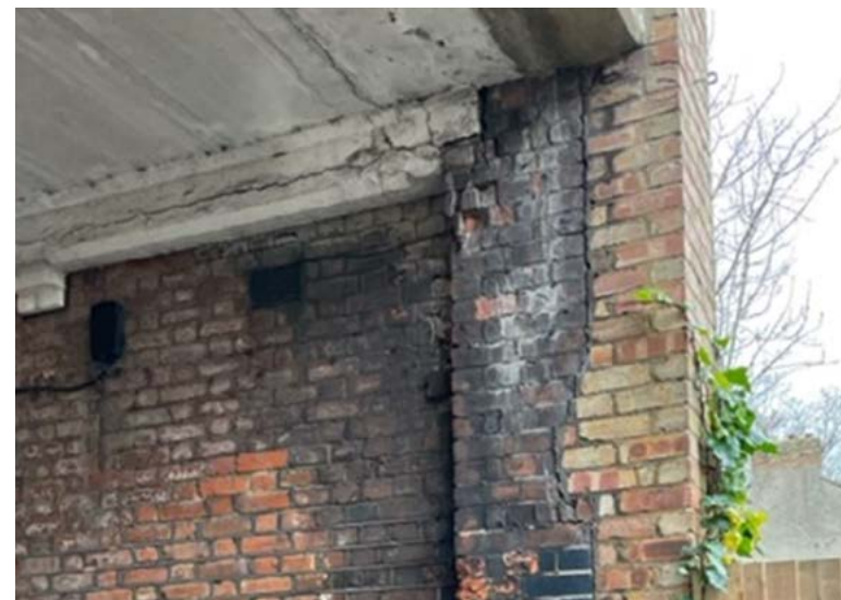
Structural deterioration in undercroft
