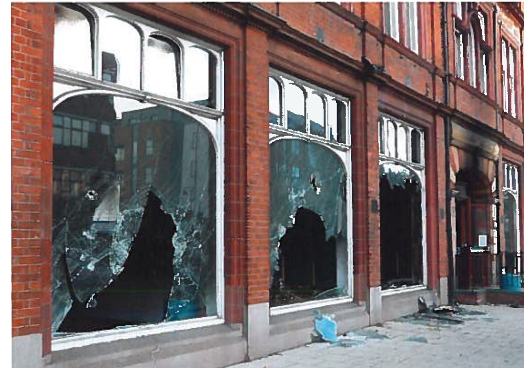
fire damaged High Road facade following the riots in 2011 image courtesy of Sergison Bates planning report HGY-2012-1561
