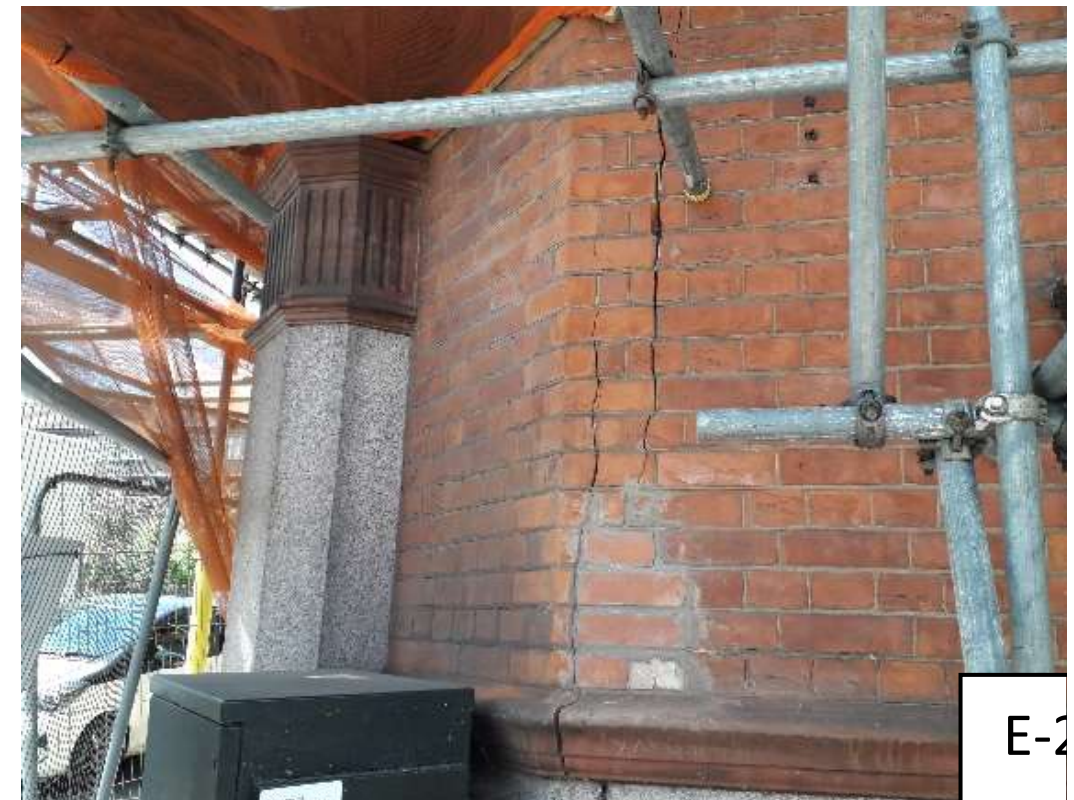
East facade crack- repairs already granted permission under HGY/2019/1968
