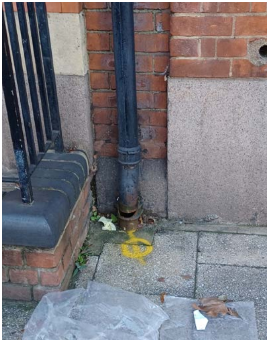
Damage to downpipe at ground level with corroding cast iron
