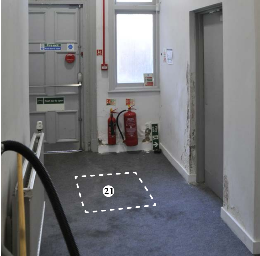
Approximate location of MH 21 to be exposed & evident water damage to walls
