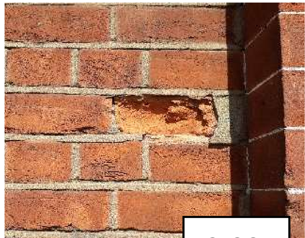
Spalling brickwork caused by cement-rich repointing
