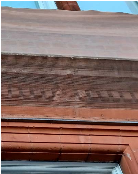
Deterioration of details to cornice dentils and profiling
