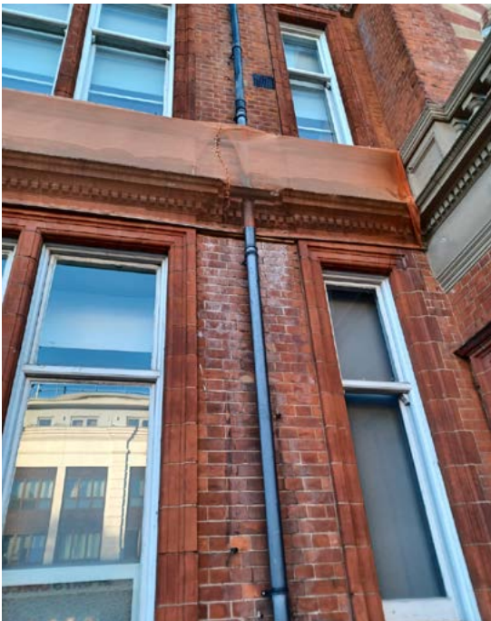
Heavy staining and deterioration of brickwork behind downpipe
