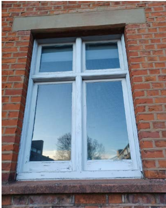
Inappropriate lintel replacement and open joints around the window
