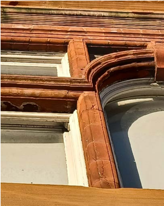
Damage to terracotta window jambs and transoms
