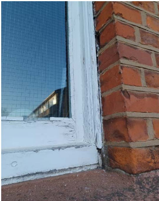
Damage to timber frame and open joints to window surround
