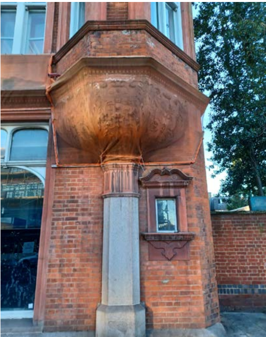
Water staining and damage to masonry
