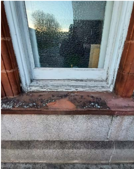
Damage to window cills and poor decoration of window frames
