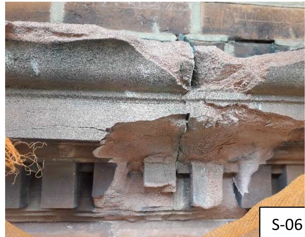
Example of decorative masonry deterioration
