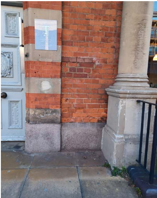
Damage to brickwork and loose mortar with cement repairs
