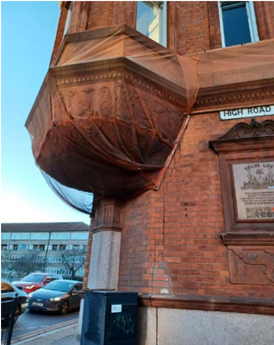
Large cracks through masonry to corner of building
