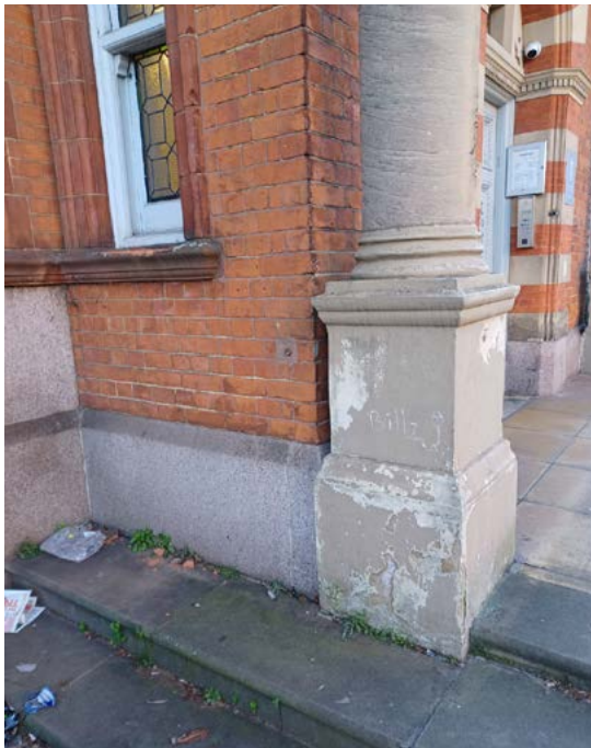
Damage to shelter coatings on stone
