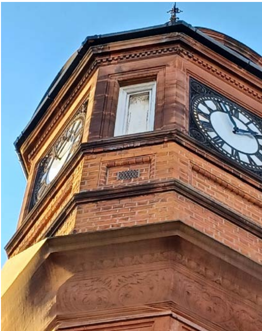
Deteriorating and rotten timber to clock tower
