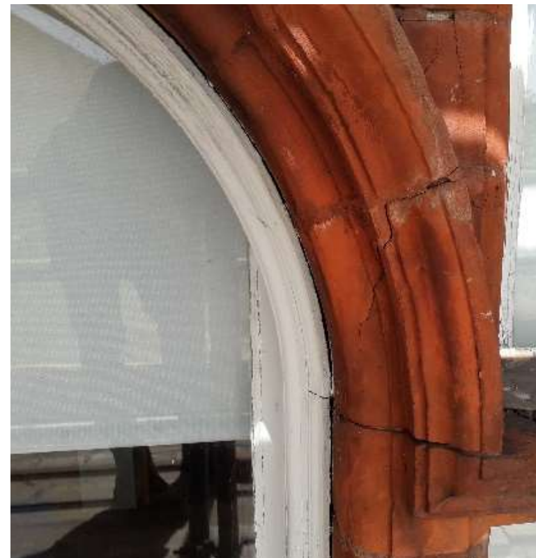
Displacement and fractures of terracotta
