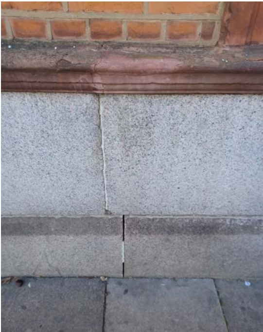
Open Joints and cracks to plinth and cement pointing
