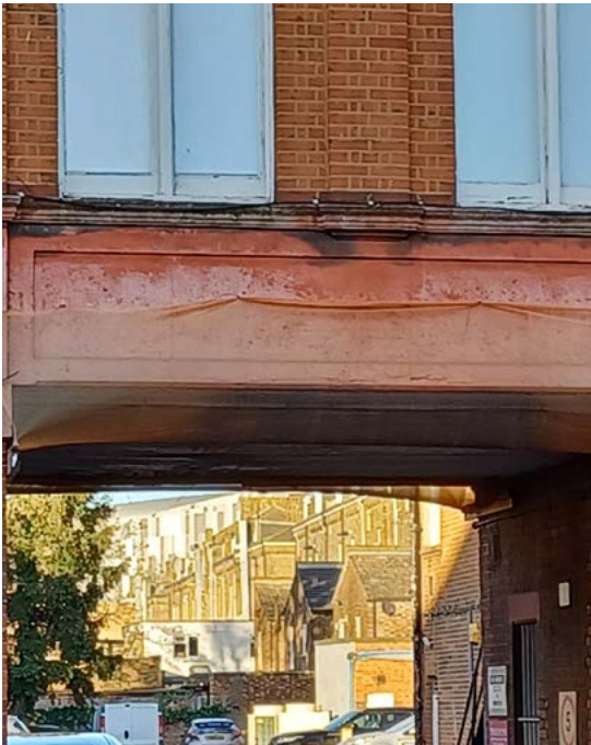
Cracked and loose render - netted for protection
