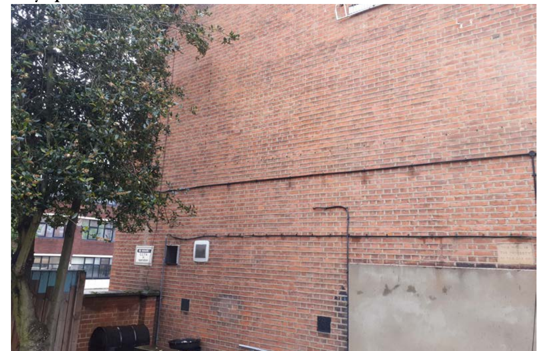
surface mounted services and conduits to the northern flank elevation
