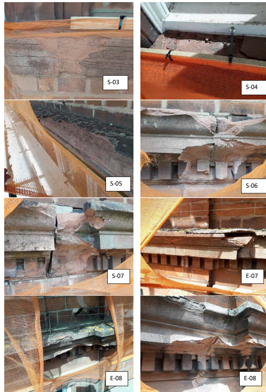
Missing pointing to L01 cornice and string course which has caused erosion or delamination of the stone. Risk of further deterioration and sections of stone falling. Note the failure of the windowsill flaunching (S-04)
