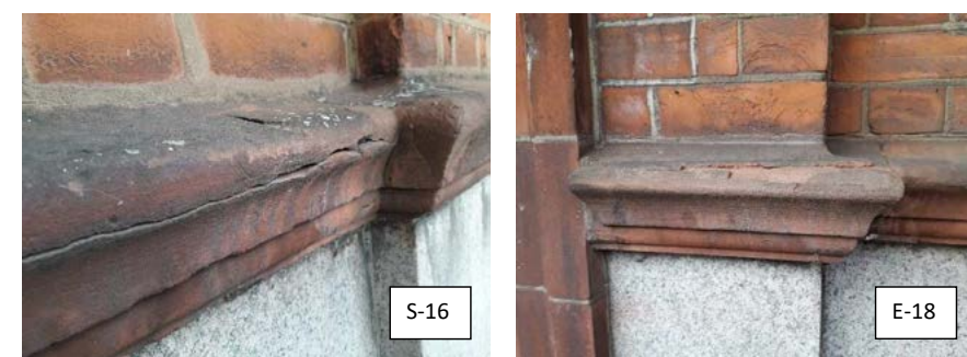
Missing pointing to L01 cornice and string course which has caused erosion or delamination of the stone. Risk of further deterioration and sections of stone falling. Note the failure of the windowsill flaunching (S-04)
