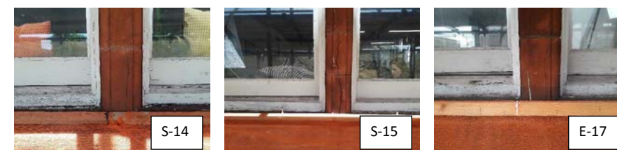
Vertical fractures observed to terracotta window mullions.
