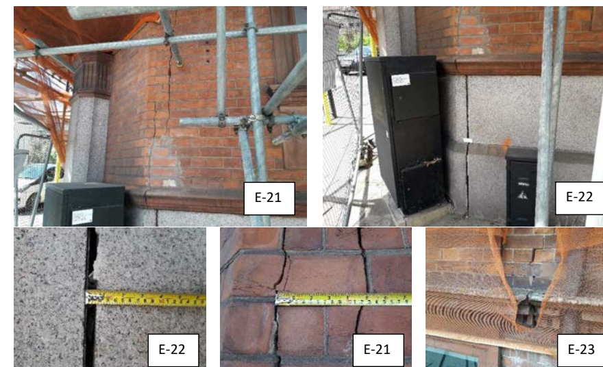
Fractures observed through brickwork to the SE corner
