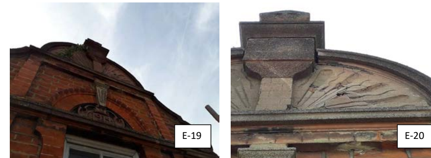
The render repair to two of the gables has blown and is at risk of falling.
