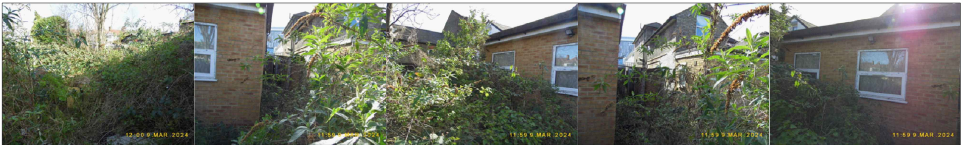
VIEW OF REAR GARDEN LOOKING TO REAR TOTALLY OVERGROWN VIEW OF REAR ELEVATION VIEW OF REAR ELEVATION LOOKING WEST VIEW OF REAR ELEVATION LOOKING EAST VIEW OF REAR ELEVATION
