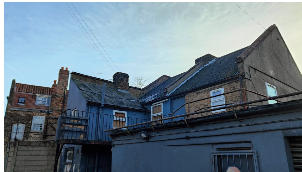
Vacant one roomed apartment with suspected asbestos roofing
