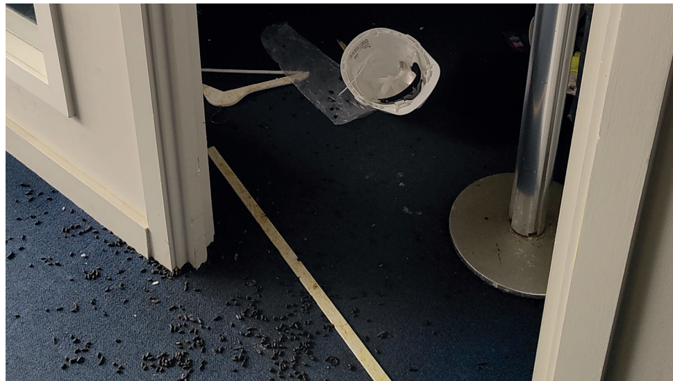
Meeting room with evidence of potential rat droppings
