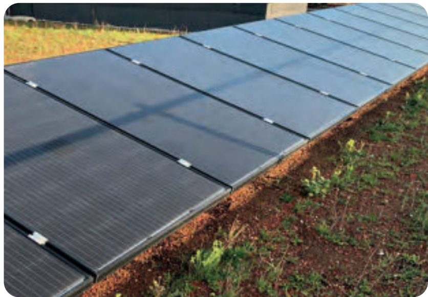
Photovoltaic Panels incorporated into a green roof
