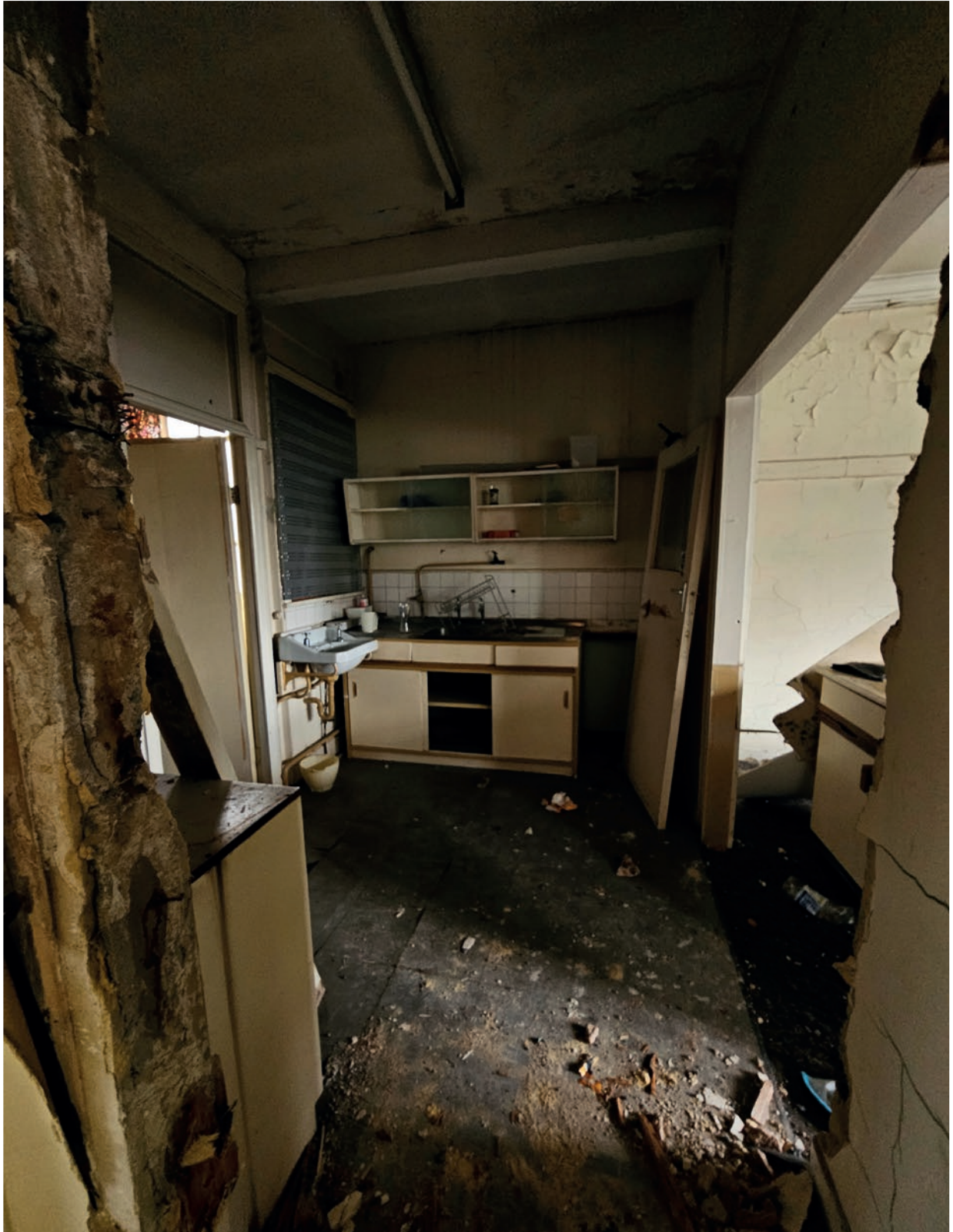
Internal view showing derelict space in poor state of repair
