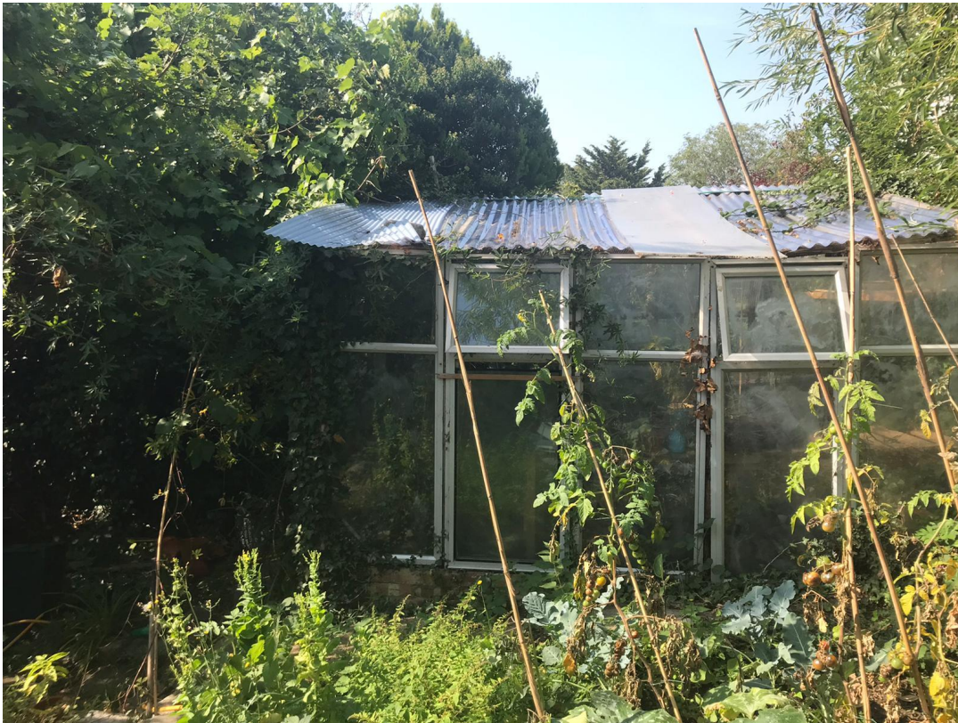
Photograph 1 – Derelict greenhouse located to the rear of 10 Bidwell Gardens.
