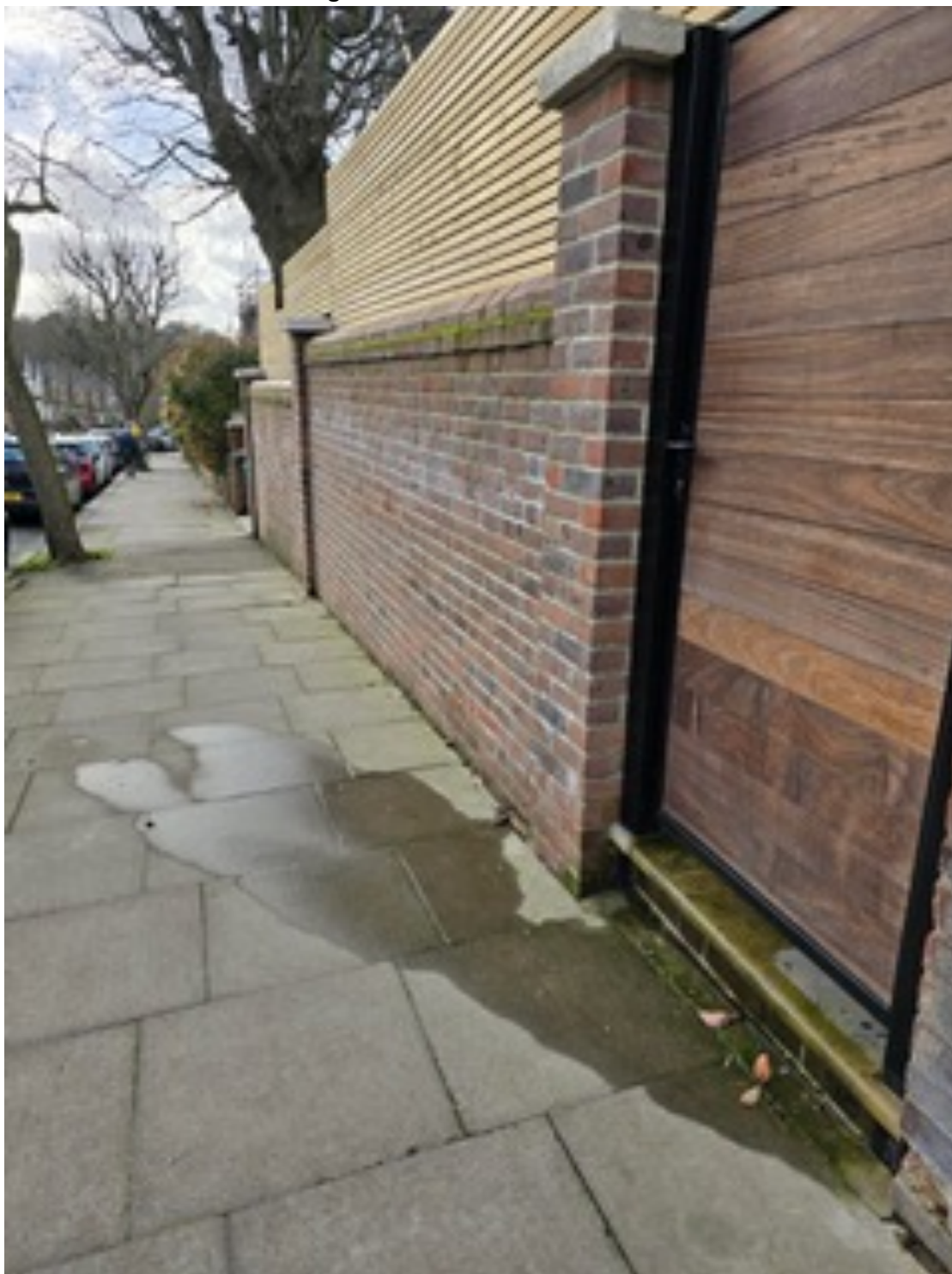
Excessive water run-off from garden of 1A The Avenue into sewers of Dukes Avenue
