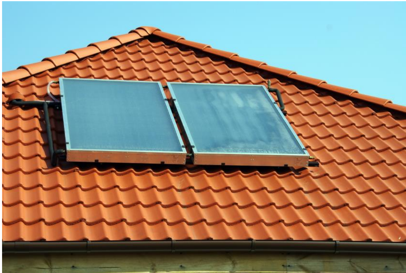
FIGURE 20 –SOLAR WATER HEATING SYSTEM
