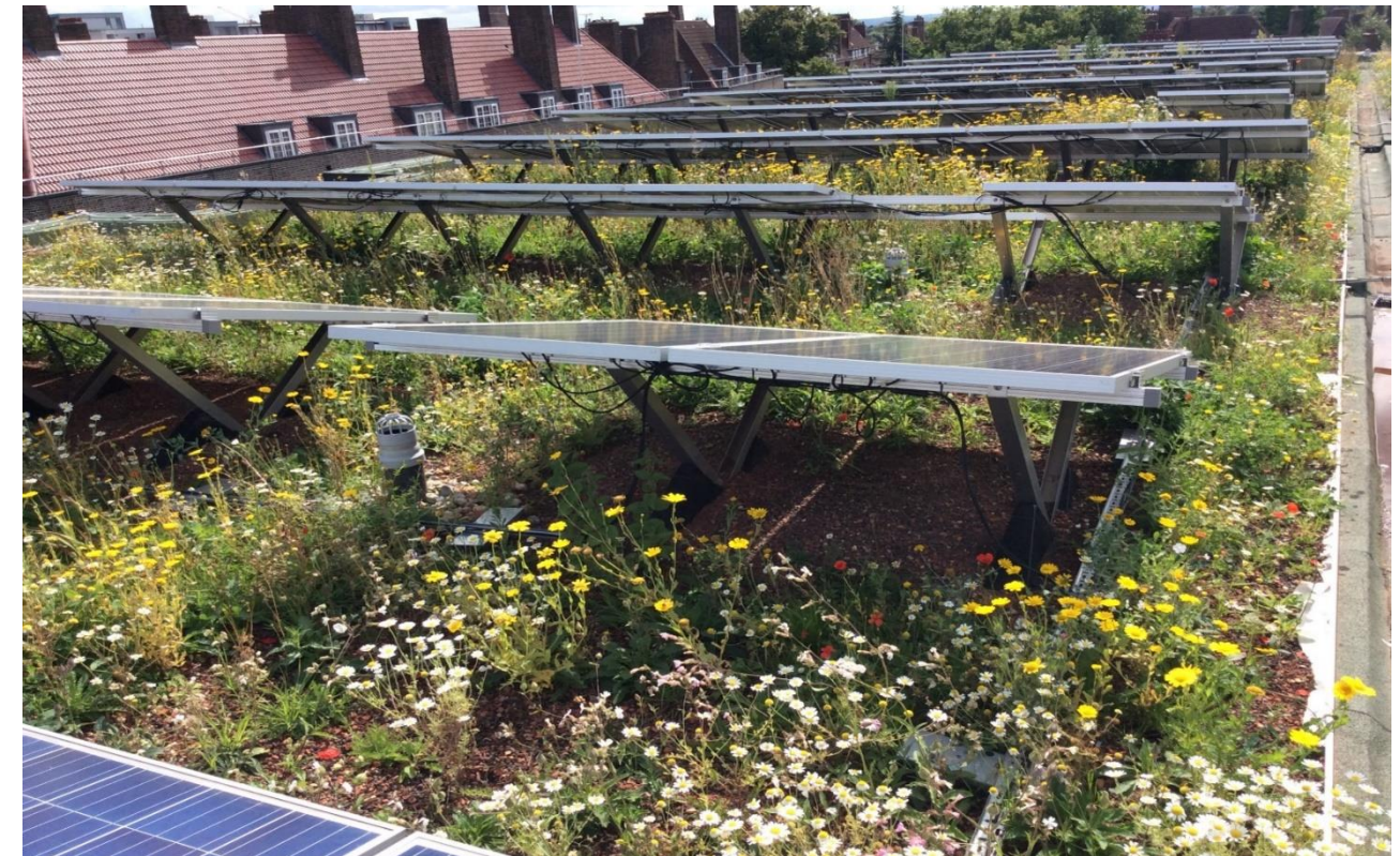
FIGURE 01 – ROOF COMBINING PV PANELS AND WILDFLOWER BLANKET
