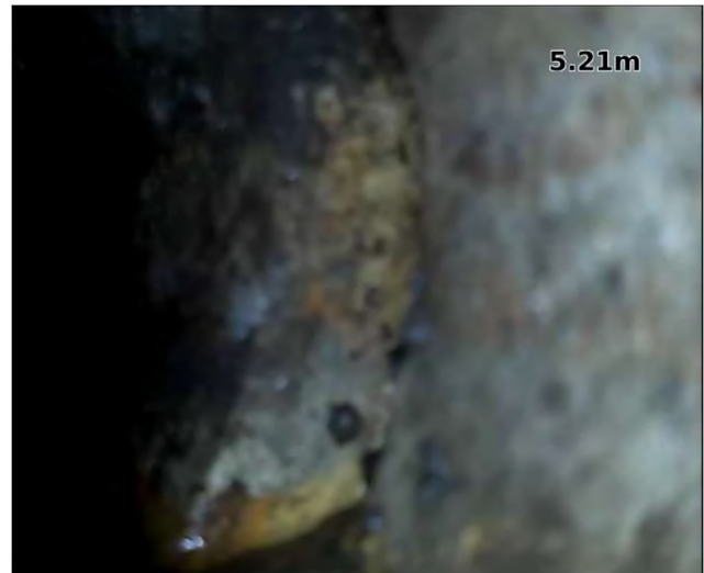
Joint Displaced Large
