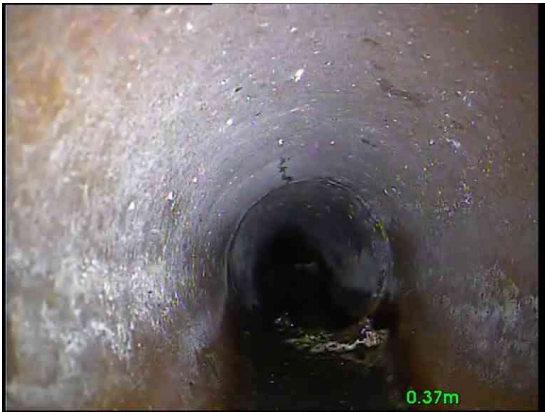
2, 00:00:05, 0.37 m Settled deposits, hard or compacted at joint, 10% cross-sectional area loss
