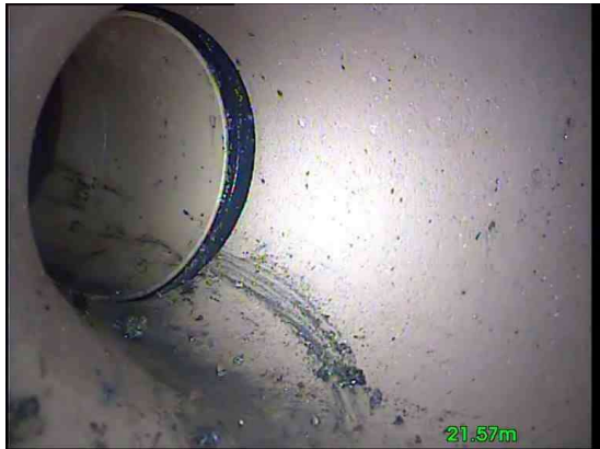
23, 00:02:27, 21.57 m Open joint, large
