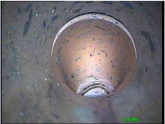
2, 00:00:09, 0.59 m Joint displaced, medium, At entry to RWP gully pot
