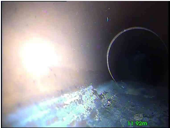
10, 00:00:57, 11.92 m Settled deposits, fine, 10% cross-sectional area loss, finish
