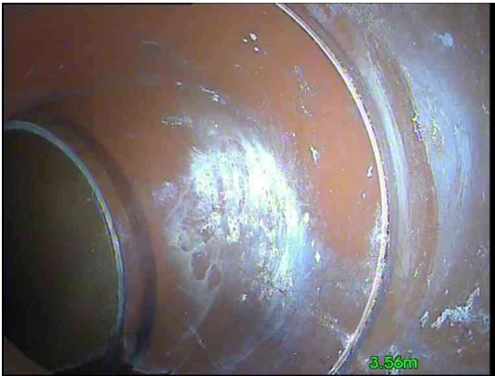
5, 00:00:17, 3.56 m Line deviates down
