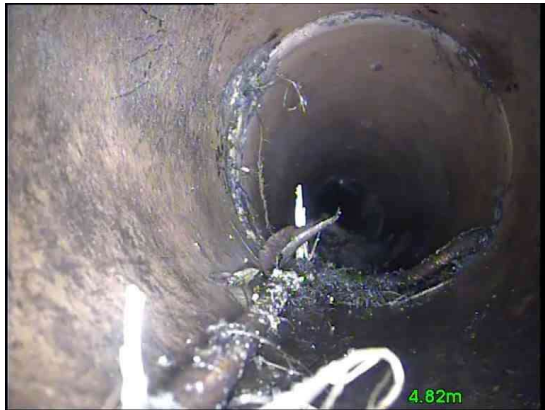
7, 00:00:45, 4.82 m Roots, tap at joint
