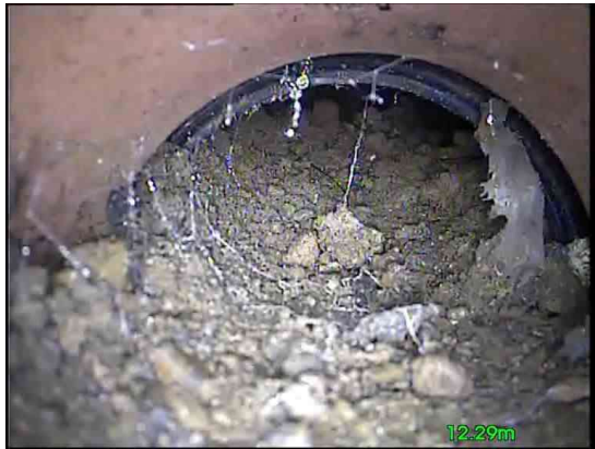
9, 00:00:53, 12.29 m Settled deposits, coarse, 75% cross-sectional area loss, change
