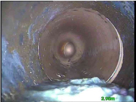
4, 00:00:26, 2.95 m Pipe material changes to polyvinyl chloride at this point
