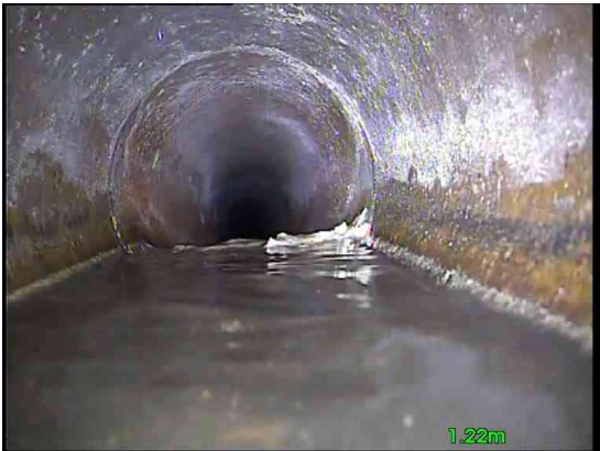
4, 00:00:10, 1.22 m Settled deposits, hard or compacted at joint, 20% cross-sectional area loss
