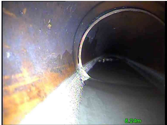
8, 00:00:40, 8.24 m Water level, 25% of the vertical dimension, Water standing in sewer at this point
