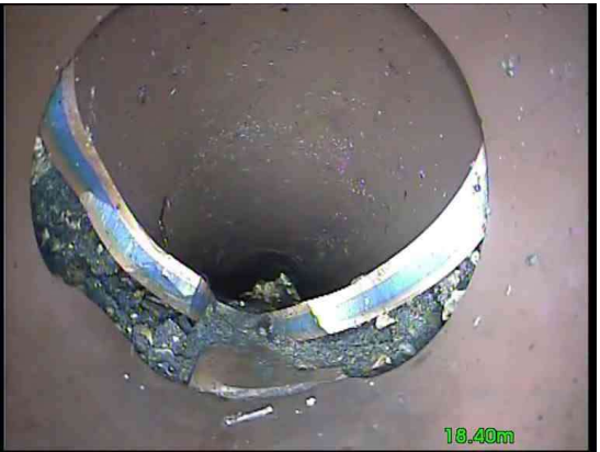
6, 00:01:09, 18.40 m Joint displaced, large
