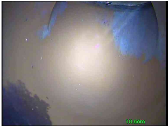
6, 00:00:47, 10.66 m Finish node, other special chamber, reference: Downpipe, Internal downpipe reached
