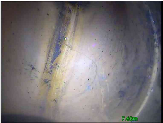
5, 00:00:54, 7.62 m Finish node, gully, reference: Gully reached
