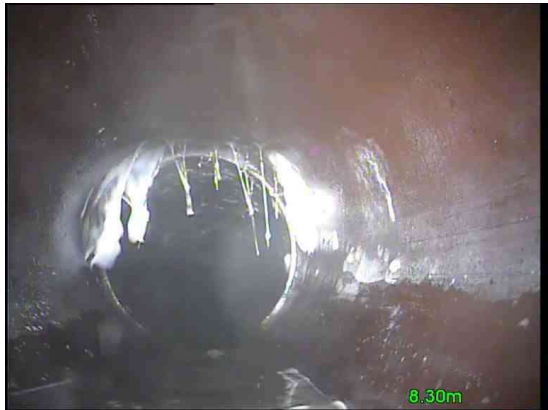
3, 00:02:23, 8.30 m Attached deposits, fouling at joint from 9 o'clock to 3 o'clock, 5% cross-sectional area loss
