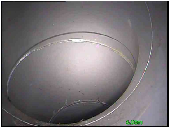
8, 00:00:50, 6.05 m General remark, Sewer levels out at this point
