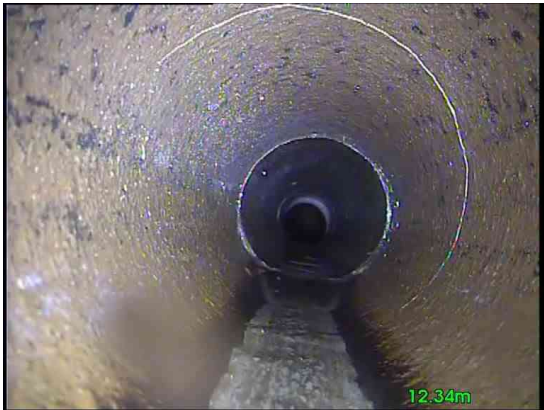
8, 00:01:00, 12.34 m Crack, circumferential from 10 o'clock to 4 o'clock
