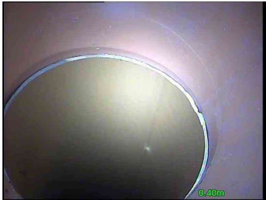
2, 00:00:10, 0.40 m General remark, Sewer levels out at this point
