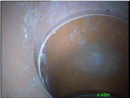
7, 00:00:34, 6.62 m Line deviates down
