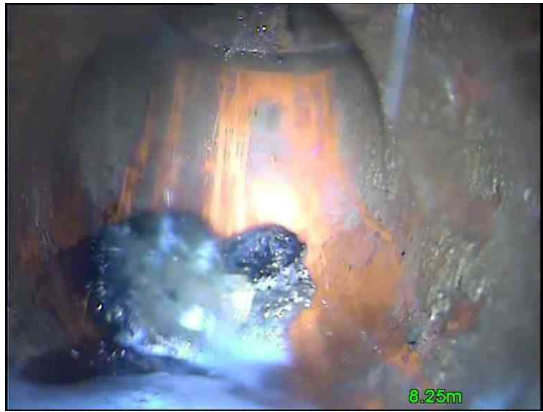
7, 00:01:18, 8.25 m Settled deposits, coarse, 5% cross-sectional area loss, At rest bend of internal downpipe
