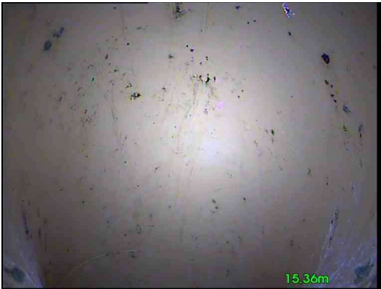
5, 00:00:44, 15.36 m Line deviates down
