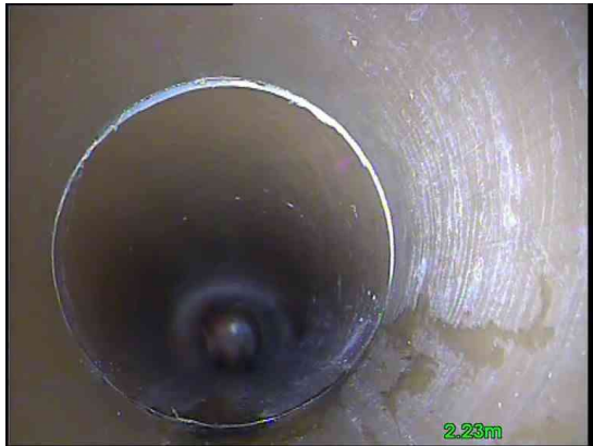
3, 00:00:13, 2.23 m Line deviates down
