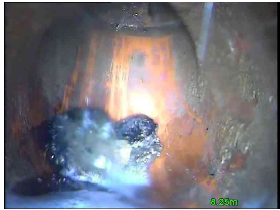
8, 00:01:18, 8.25 m Finish node, other special chamber, reference: Downpipe, Internal downpipe reached
