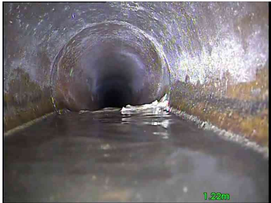
3, 00:00:10, 1.22 m Water level, 20% of the vertical dimension, Water standing due to debris at joint
