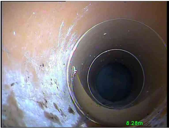
4, 00:00:38, 8.28 m Junction at 6 o'clock, 150mm dia, External Backdrop
