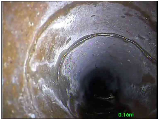
1, 00:00:03, 0.16 m Crack, circumferential from 9 o'clock to 3 o'clock
