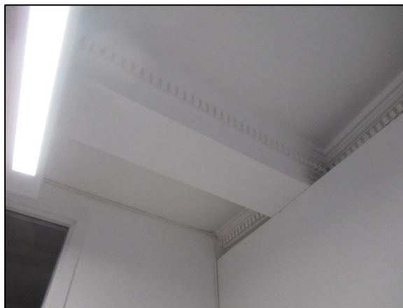
Figure 18: Room 1 – Obstructed Beam &amp; Cornice
