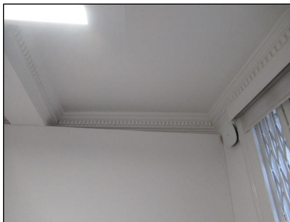
Figure 15: Room 1 – Obstructed Cornice
