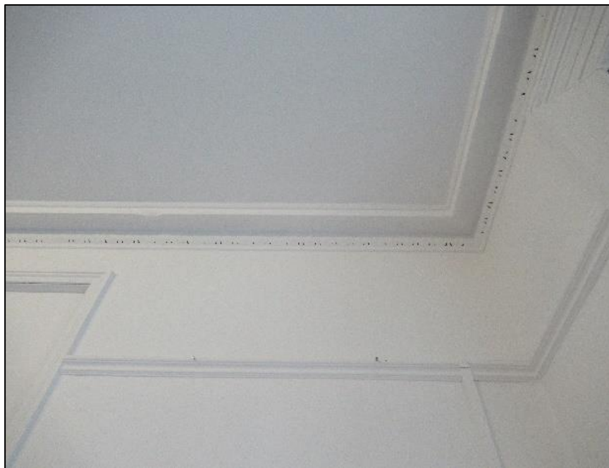
Figure 23: Painted Over Cornice
