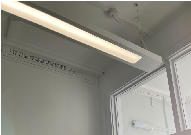
Fig. 17 - Level 0 - Section of decorative cornice missing
