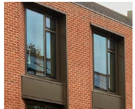
Fig. 22. Coated aluminium windows
