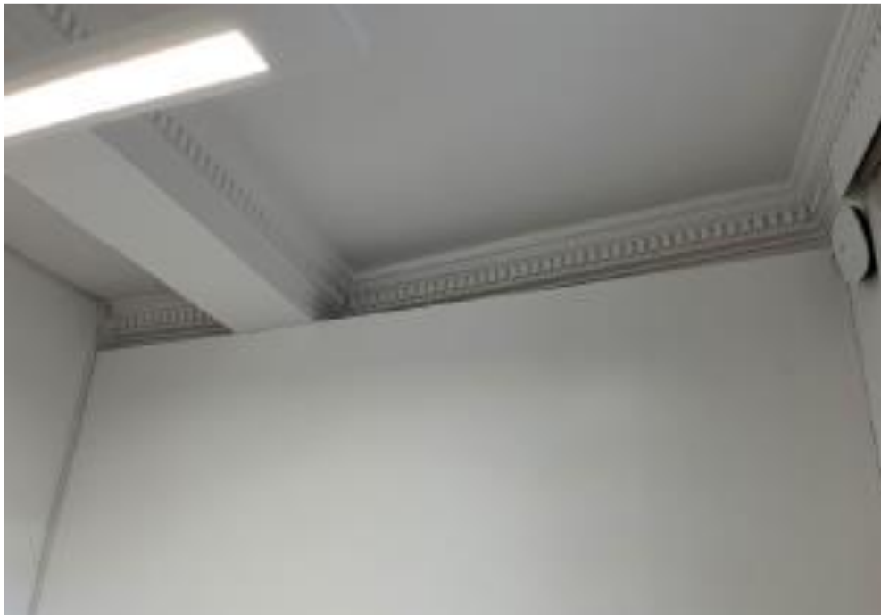
Typical example of cornicing interrupted by modern partition
