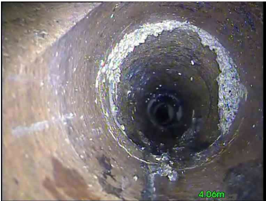
7, 00:00:35, 4.06 m Crack, circumferential at joint from 4 o'clock to 8 o'clock
