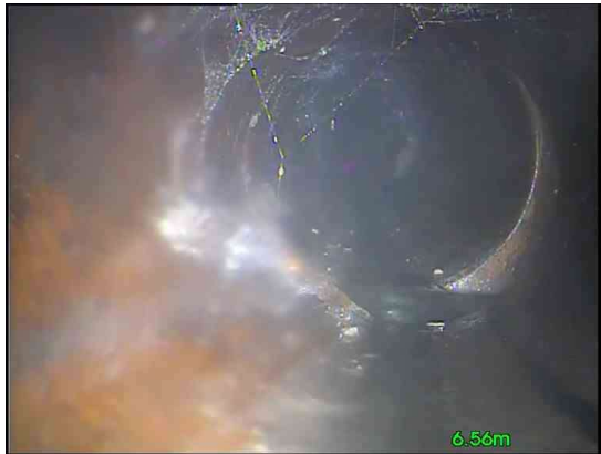
7, 00:05:01, 6.56 m Joint displaced, large
