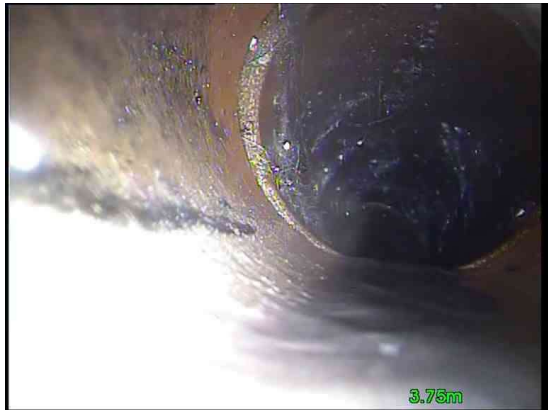
4, 00:01:03, 3.75 m Line deviates down
