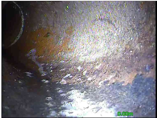
1, 00:00:02, 0.00 m Line deviates up
