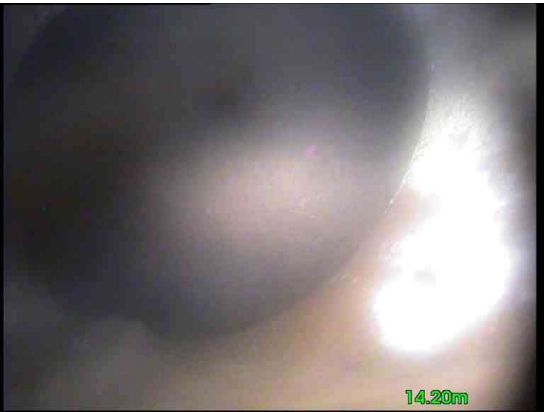
6, 00:01:07, 14.20 m Finish node, major connection without manhole, reference: Main public sewer reached
