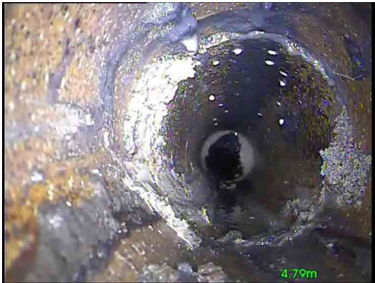
8, 00:00:39, 4.79 m Settled deposits, fine at joint, 5% cross-sectional area loss
