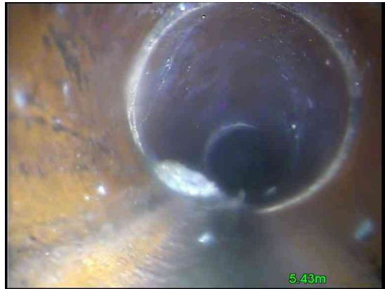
6, 00:02:48, 5.43 m Settled deposits, hard or compacted at joint, 5% cross-sectional area loss
