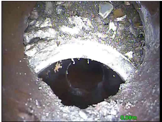
1, 00:00:05, 0.08 m Joint displaced, large
