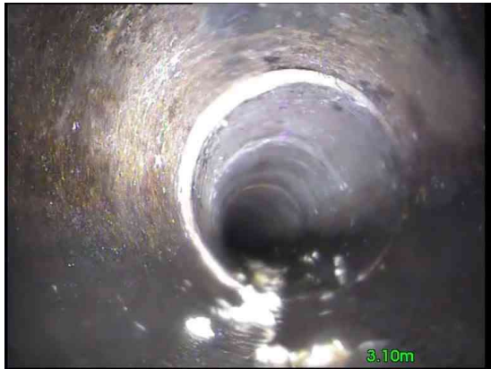
2, 00:03:45, 3.10 m Pipe material changes to vitrified clay at this point
