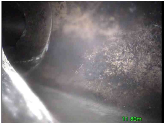
7, 00:01:10, 11.80 m Finish node, major connection without manhole, reference: Main public sewer reached
