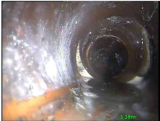
3, 00:00:51, 3.38 m Joint displaced, large
