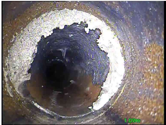
2, 00:00:11, 1.09 m Settled deposits, fine at joint, 10% cross-sectional area loss
