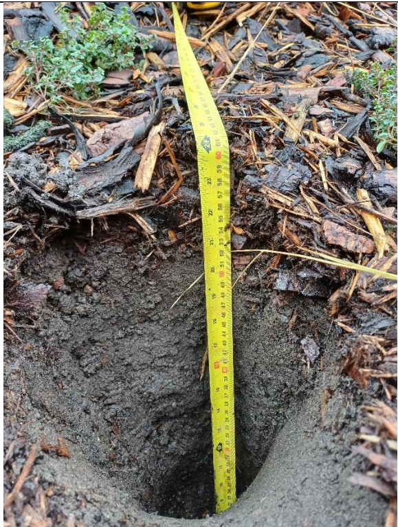
Plate 6: Roof level planter – clean cover thickness.
