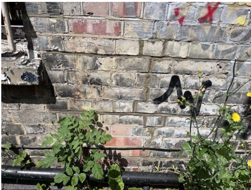
Photo 12 - Side Elevation (SE) movement and repointing at side of arched window
