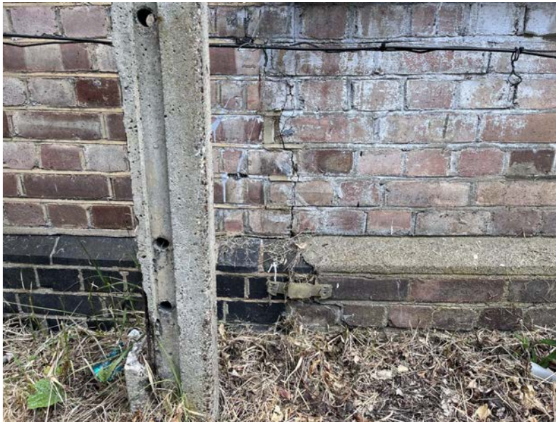
Photo 7 – Front Elevation Subsidence crack – note previously installed tell-tale monitoring
