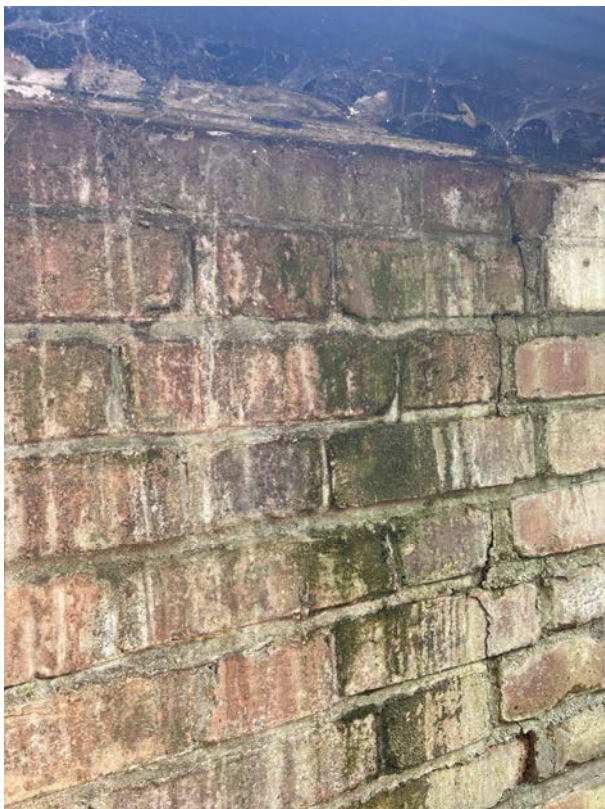
Photo 16 - Rear (NE) Elevation showing movement and cracking at eaves
