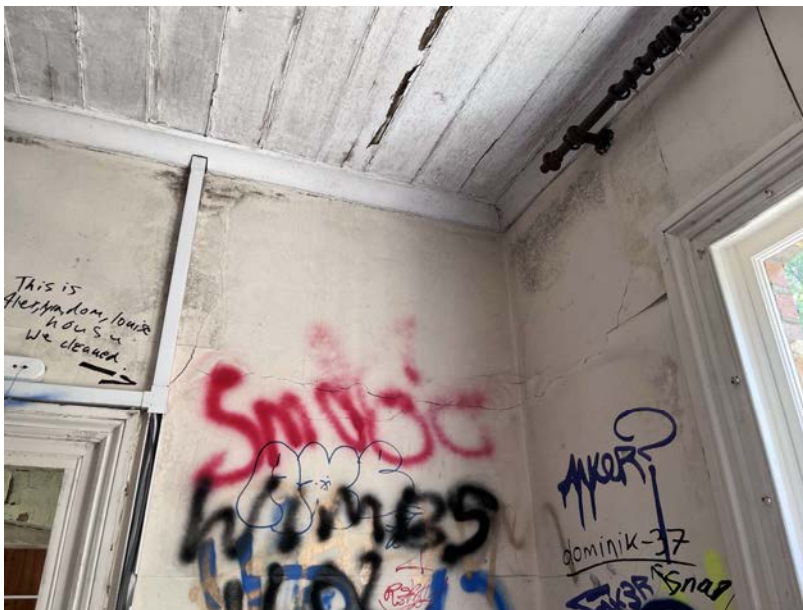
Photo 26 - Internal room off kitchen area showing vertical and horizontal cracking of wall/s
