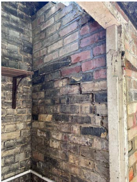
Photo 14 – Rear (NE) Elevation lean-to buttressing wall showing stepped cracking
