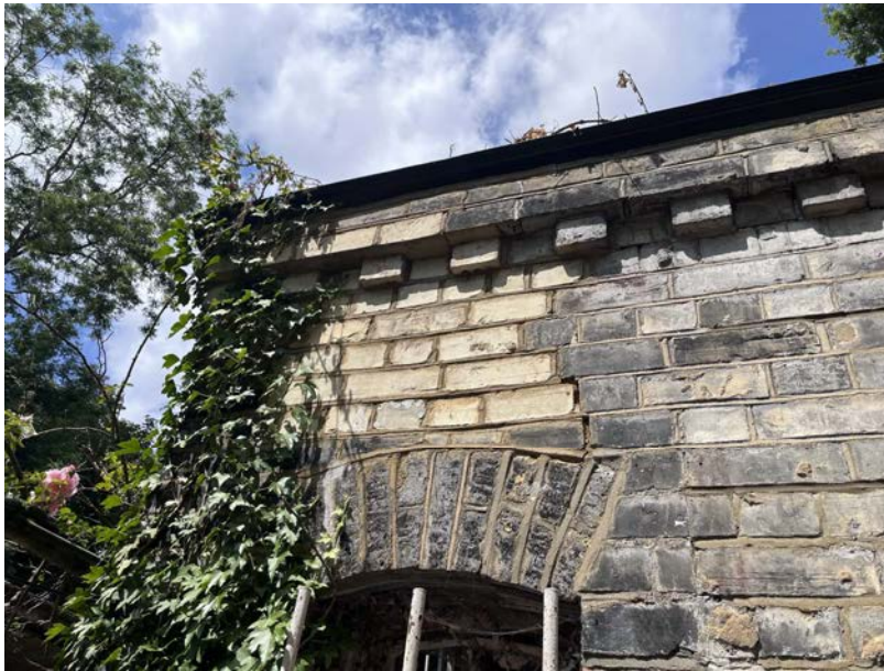
Photo 11 - Side Elevation (SE) movement and rebuilding across top of arched window (note movement still occurring)
