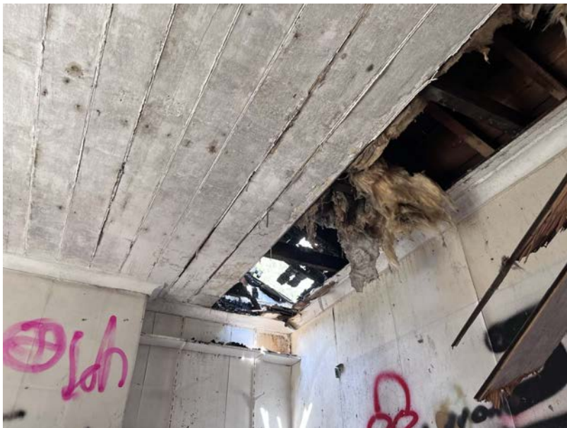
Photo 24 – Internal room off kitchen area showing damage to existing cut roof members
