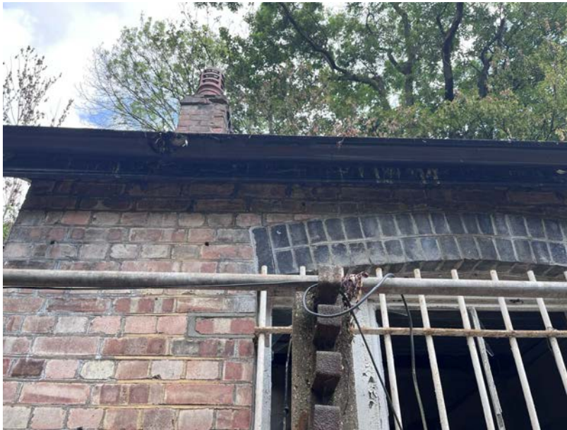
Photo 5 – Front Elevation movement over top of arched window
