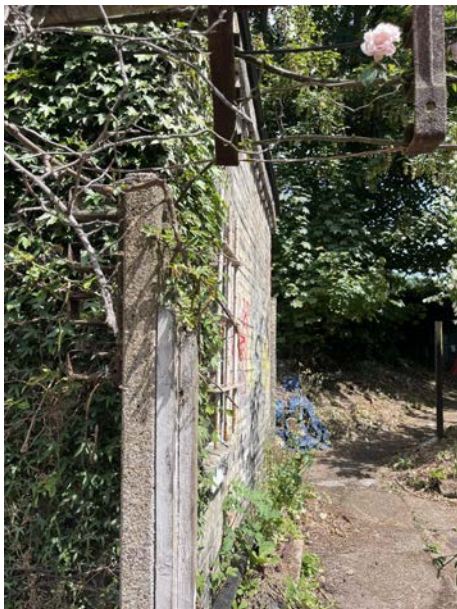
Photo 10 – Side Elevation (SE) – out of plumb wall
