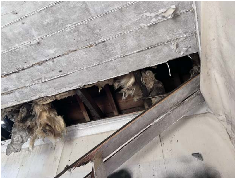
Photo 25 - Internal room off kitchen area showing damage to existing cut roof members
