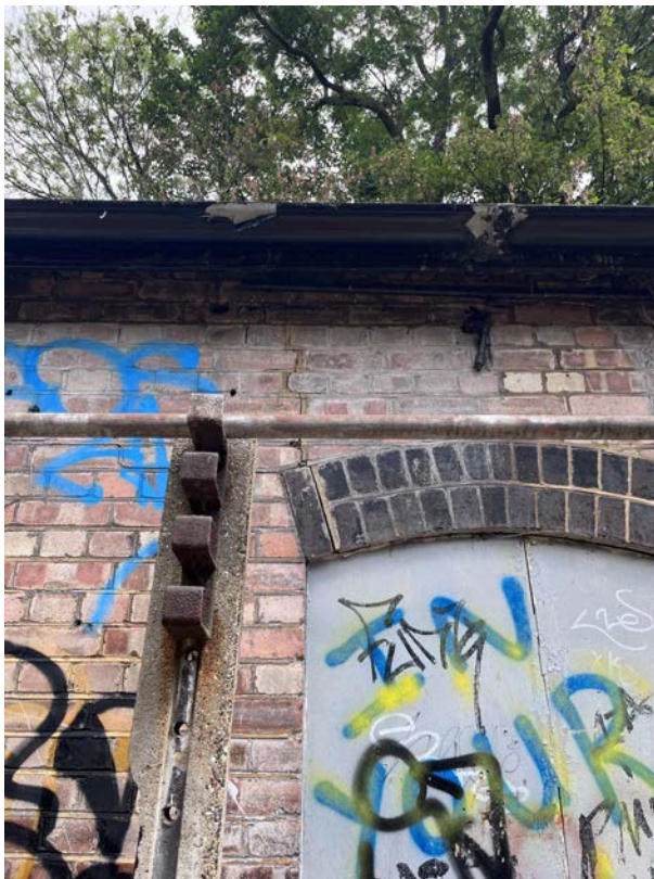
Photo 8 - Front Elevation movement over top of arched window
