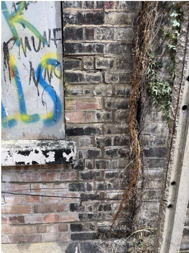
Photo 9 - Front Elevation movement and repointing to RHS of window
