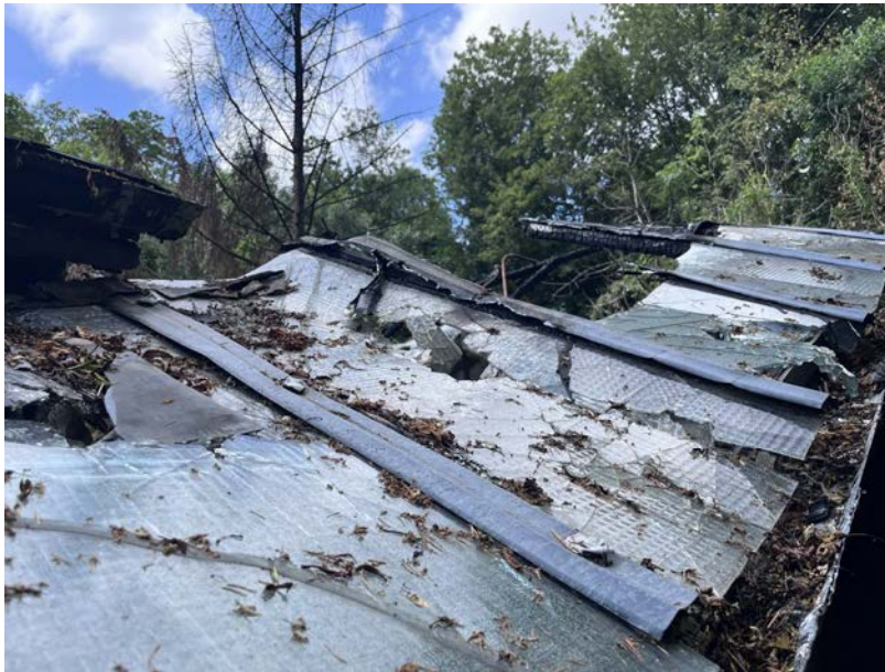
Photo 19 - Rear Elevation lean-to roof in poor condition
