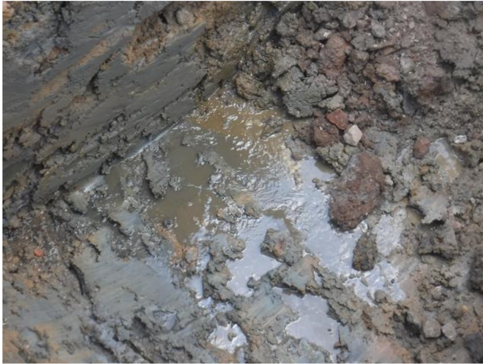
Water ingress at 3.00m.
