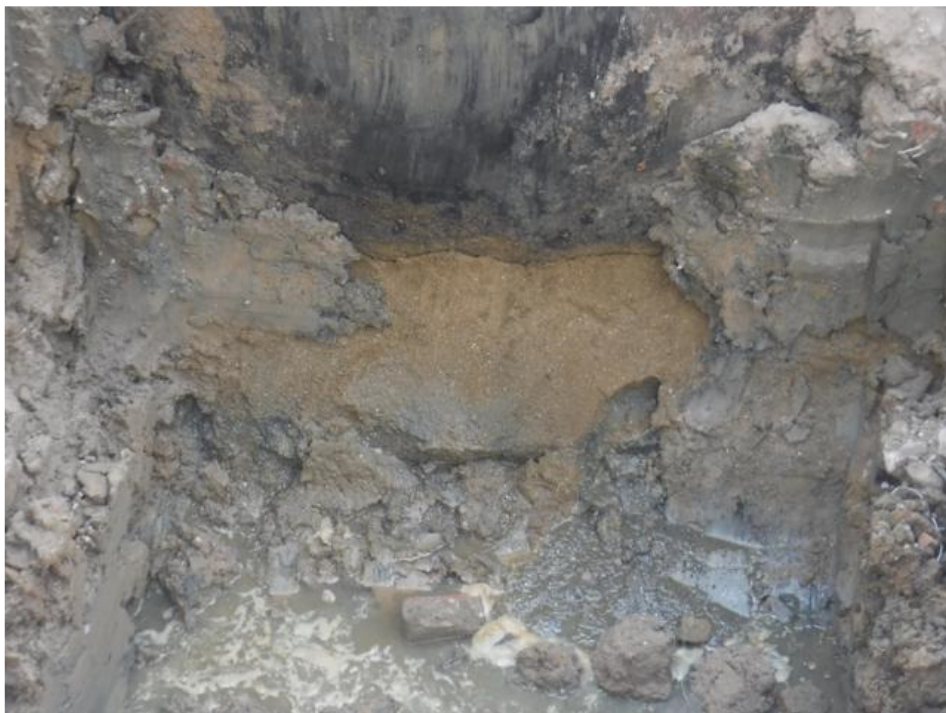
Brown sand at the base of Tank 4.
