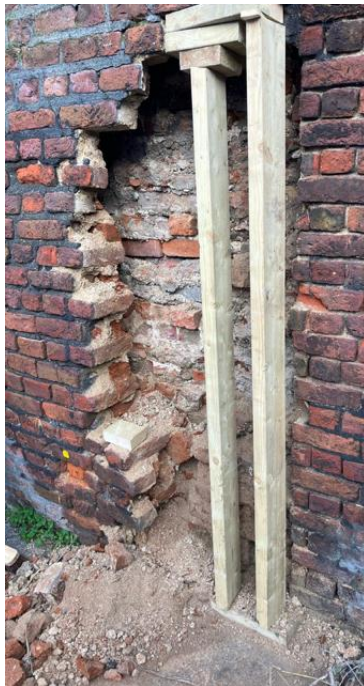
Image 9: Snapping of header causing an area of collapse
