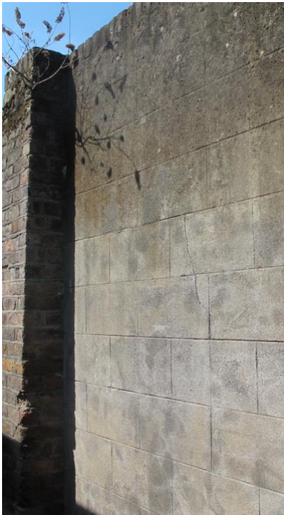
Image 6: Horizontal crack on render at approximately half its height to all bays of the wall.
