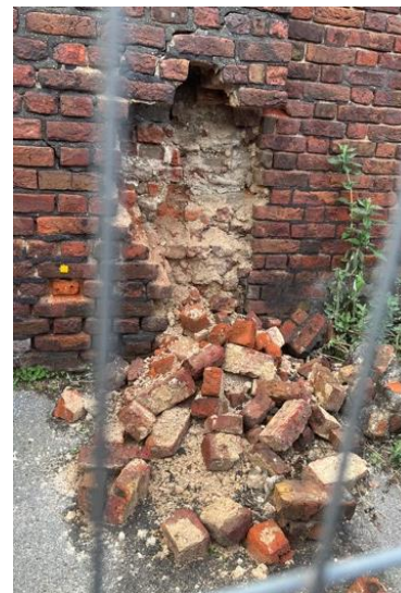
Image 1: Minor area of collapse
