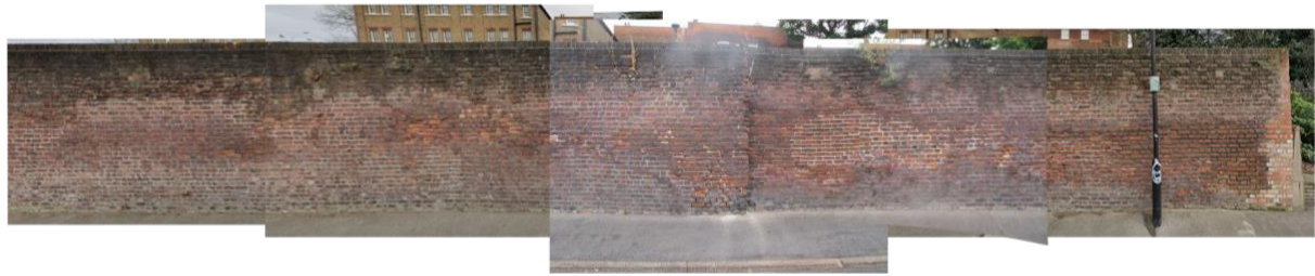
Image 12: Photographic elevation showing water damage.
