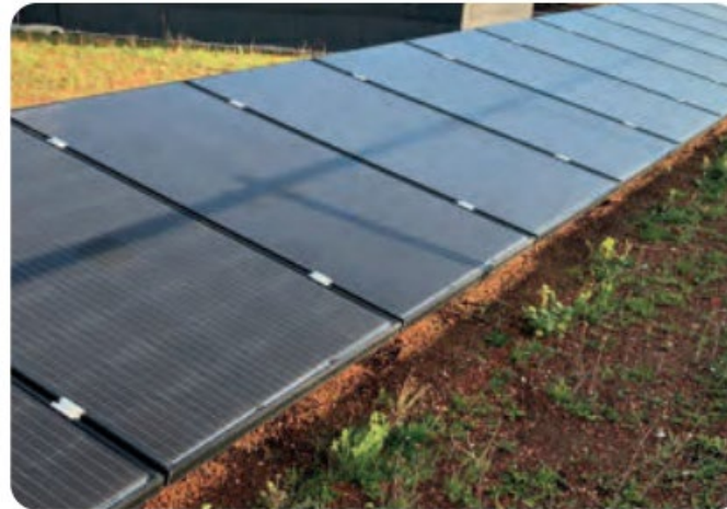
Photovoltaic Panels incorporated into a green roof
