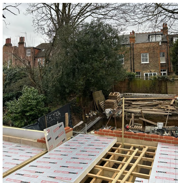
Photo taken from the first floor rear window of the property.
