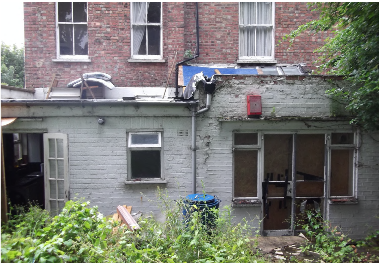
Fig.3 The existing rear addition is poorly constructed and in a poor state or repair.
