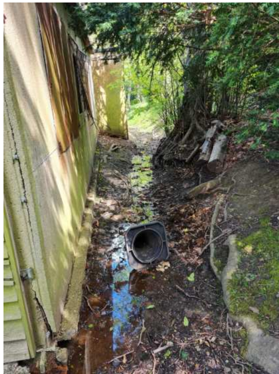
Figure 2.7: Existing ditch to the rear of the rifle range requiring clearance and improvements to increase capacity.
