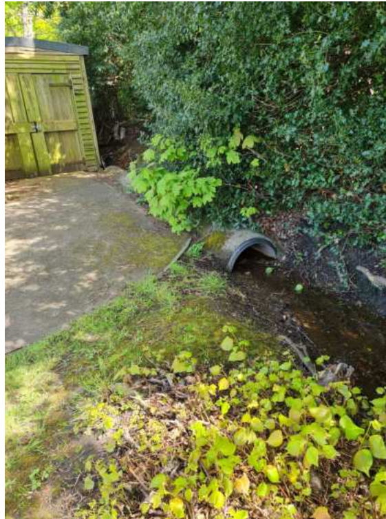
Figure 2.6: Existing culvert to the rear of the rifle range requiring jetting.
