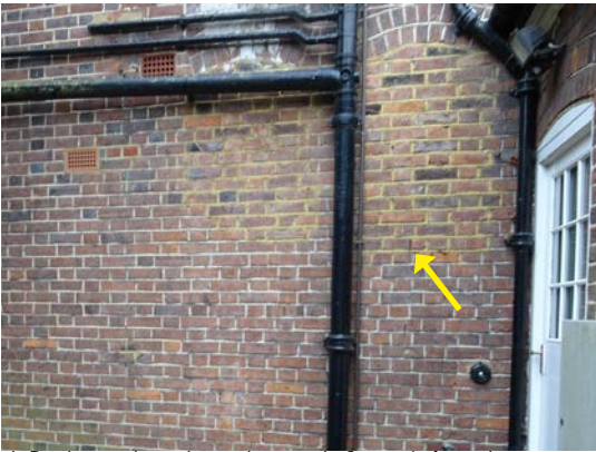
d. Brick patchwork on the north & south facades.
