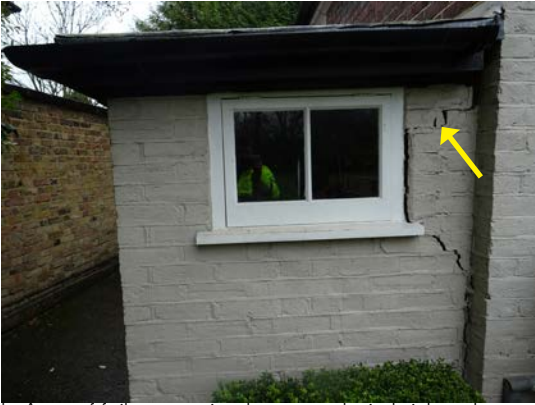
k. Area of failure causing large cracks in brickwork.
