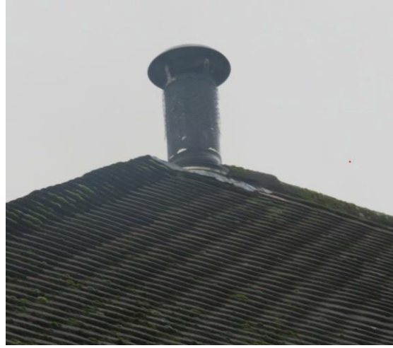
Metal flue pipe
