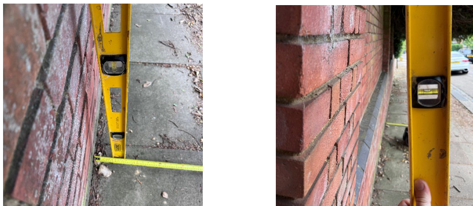
Figure 4 & 5 – Base of Wall Misalignment
