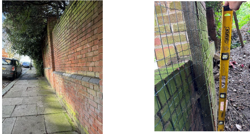
Figure 3 & 4 – Vertical lean for Later sections of Boundary Wall
