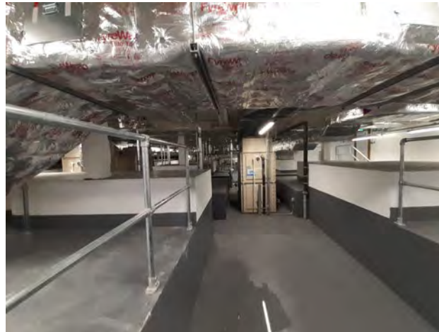
65A LG.43 Plant Room beneath Assembly Hall 2
