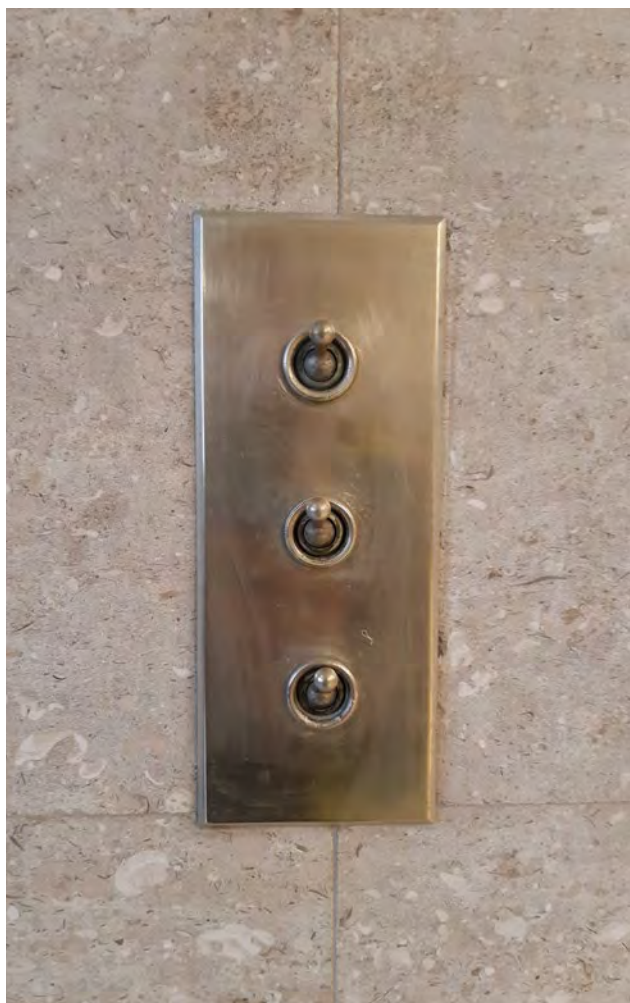
85E G.41 Entrance Hall light switches
