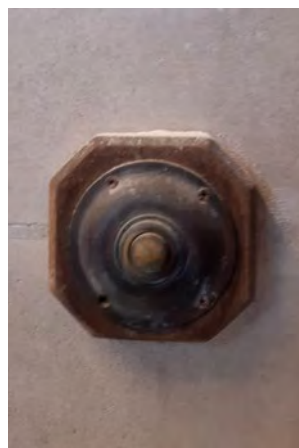
44D original light switches
