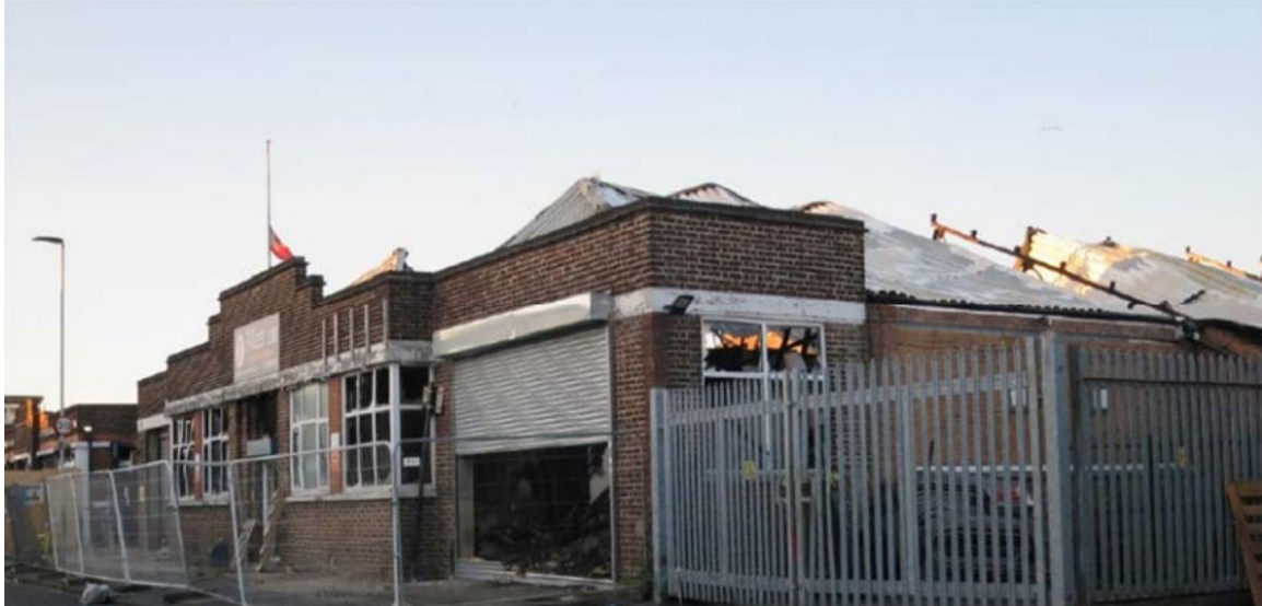
Image 4: Photograph of Fire Damage Unit June 2019
