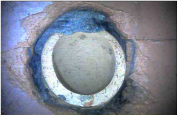
Connection other than junction at 12 7.03m, diameter: 100mm
