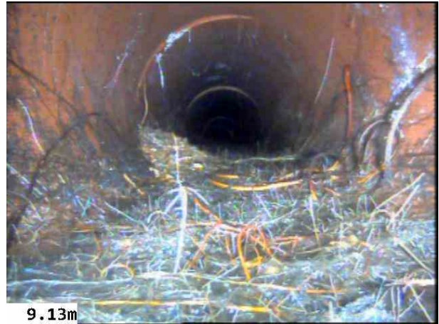
Garden 1X_a6664f8a-d5d2-485e-9306-ae7d85adfb9a_20210608_220203_442.jpg, 00:08:25, 9.13 m Survey abandoned, survey abandoned due to crawler unable to get pass debris
