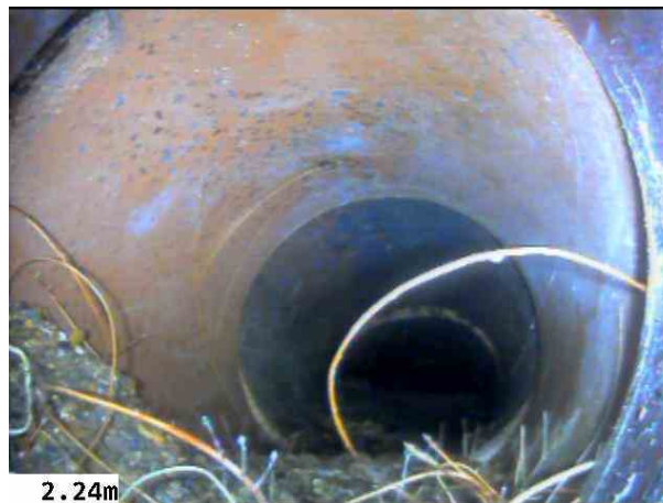
Garden 1X_dd4cb79b-82fb-4b5c-800c-06b83d48be8d_20210608_215 203_709.jpg, 00:01:29, 2.24 m Connection other than junction at 3 o'clock, diameter: 300mm, connection
