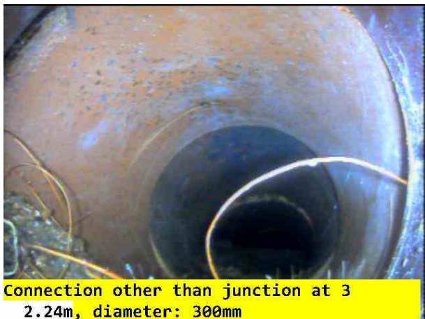
Garden 1X_d04540f9-b93c-4312-8144-1464a774e2c5_20210608_215 200_630.jpg, 00:01:29, 2.24 m Connection other than junction at 3 o'clock, diameter: 300mm, connection
