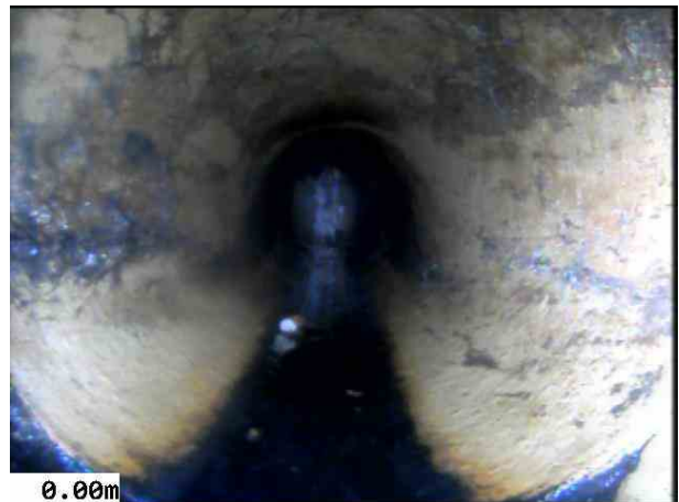
Prop MH2X_4a6eaf6a-dd9a-4830-9109-8b711409eb4a_20210608_ 223354_478.jpg, 00:08:25, 0.00 m Water level, 5% of the vertical dimension, live flowing water
