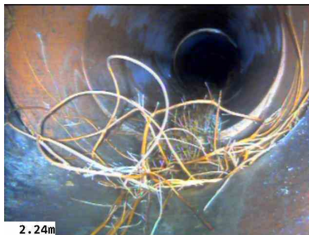
Garden 1X_4517b416-12e5-4861-985b-eae0c8bead6b_20210608_215 255_277.jpg, 00:01:45, 2.24 m Roots, fine at joint, fine roots in joint
