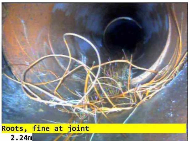
Garden 1X_bfc166f0-2869-4cab-ba87-cd3921366bdd_20210608_2152 51_765.jpg, 00:01:45, 2.24 m Roots, fine at joint, fine roots in joint
