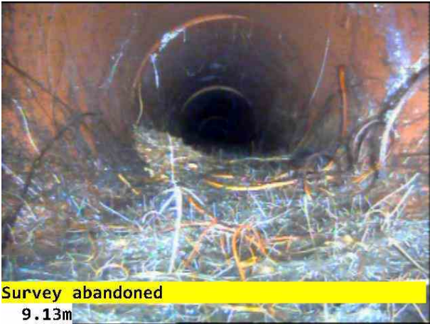
Garden 1X_fc882bd2-6db1-48c2-99b8-78ec3c304a44_20210608_220154_280.jpg, 00:08:25, 9.13 m Survey abandoned, survey abandoned due to crawler unable to get pass debris
