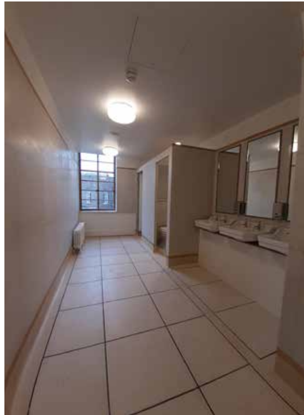
118 F.41 Men's Lavatory
