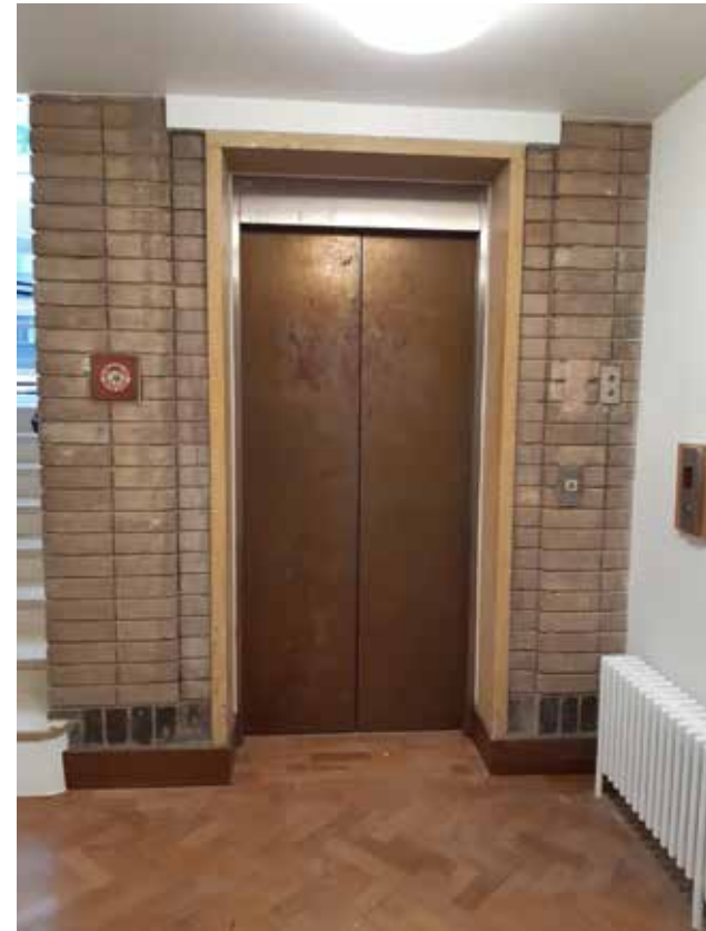
50B lift doors
