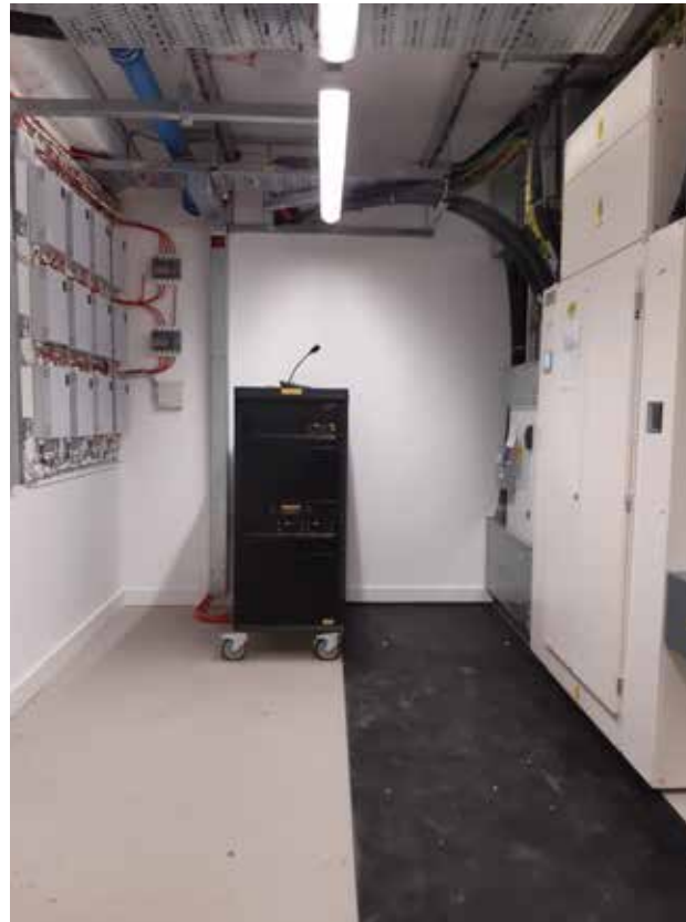
51 LG.5c Switch Room
