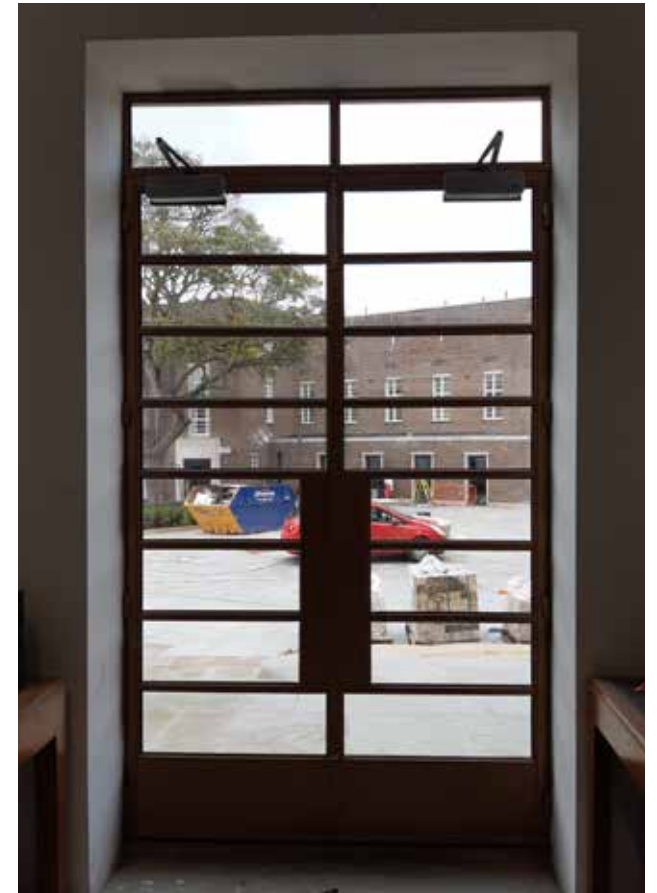
81D G.38 F&B Restaurant doors (new double glazed)
