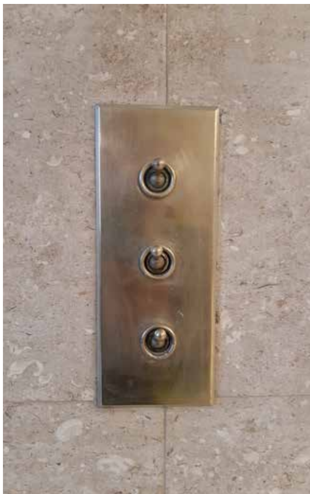
85E G.41 Entrance Hall light switches
