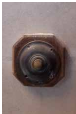
44D original light switches
