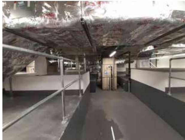
65A LG.43 Plant Room beneath Assembly Hall 2
