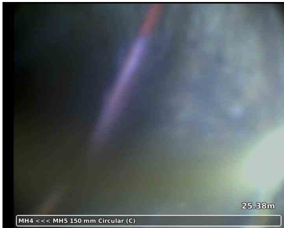
20240514-113115-snap0000.jpg, 00:03:21, 25.38 m Large displaced joint
