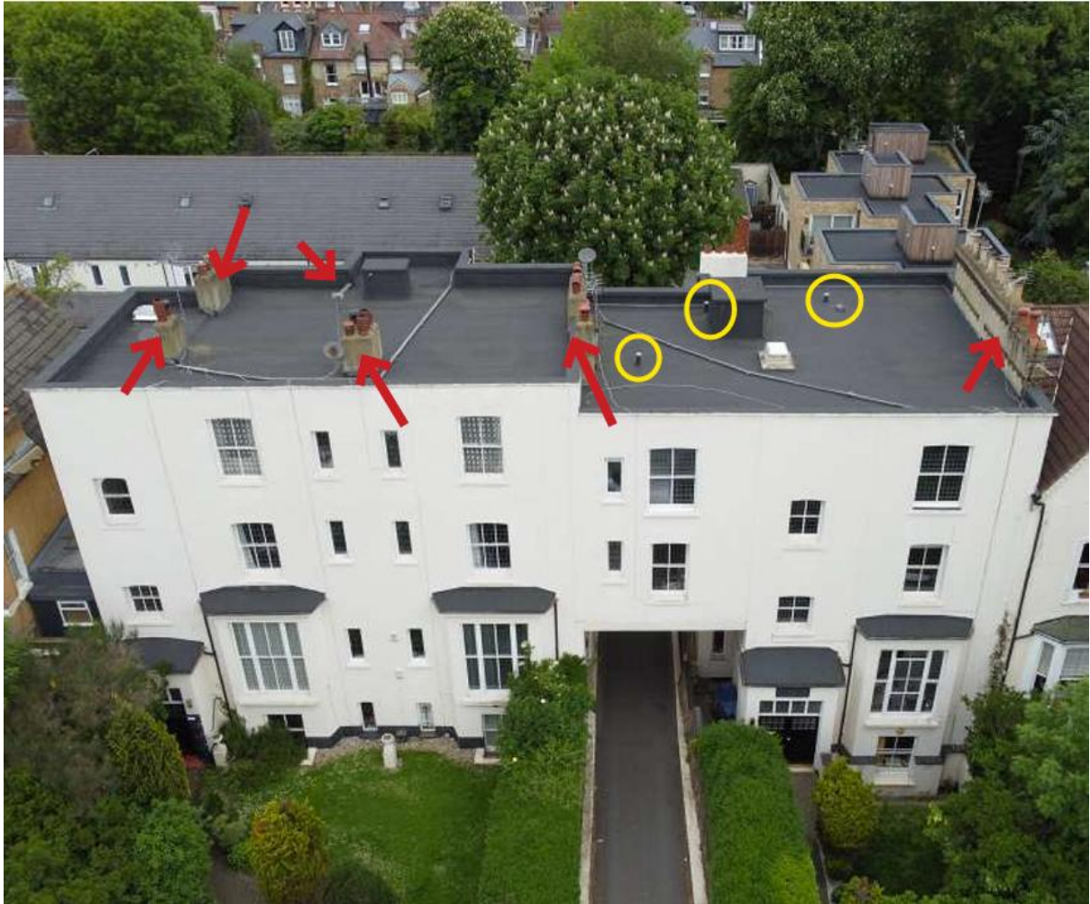
Ventilation and extraction circled in yellow.
