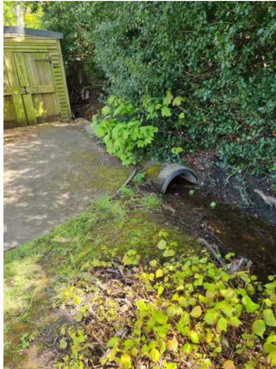
Figure 2.4: Existing culvert to the rear of the rifle range requiring jetting.
