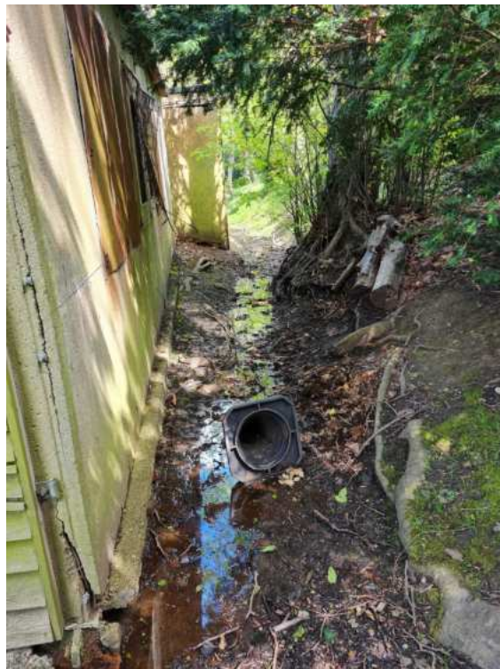
Figure 2.5: Existing ditch to the rear of the rifle range requiring clearance and improvements to increase capacity.
