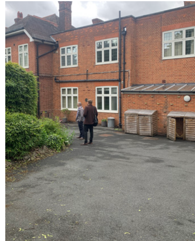
Unsympathetic extension to Kekewich House.
