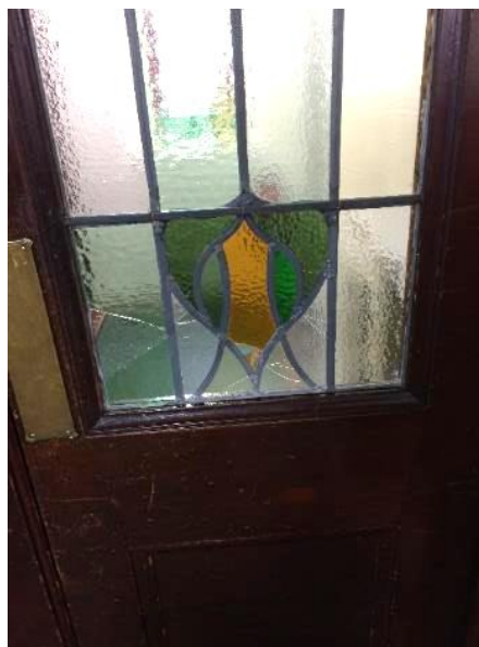
Figure 4.11: Cracking to stained glass windows.
