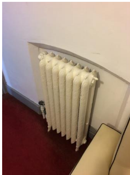
Figure 4.25: Decorative cast iron radiators.
