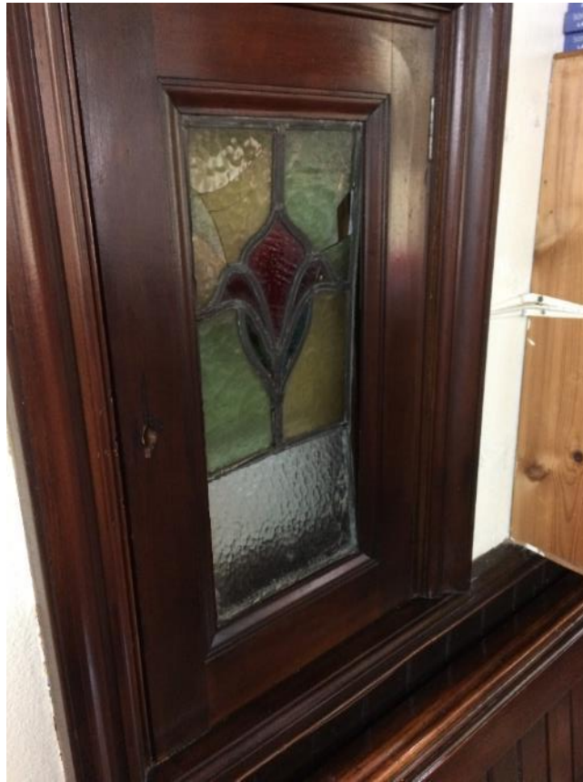
Figure 4.12: Bowing stained glass window close to entrance vestibule.
