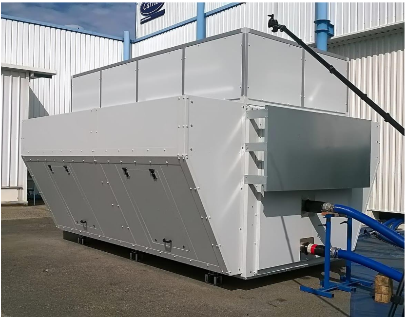
Figure 6—5 Chiller attenuation package
