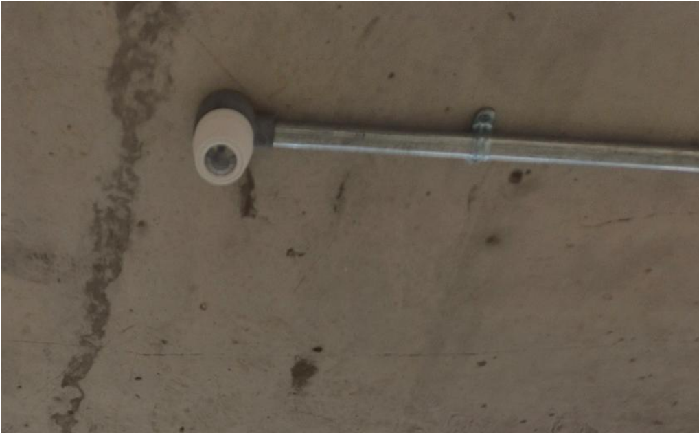
PIR controls the lighting in the bin store.
