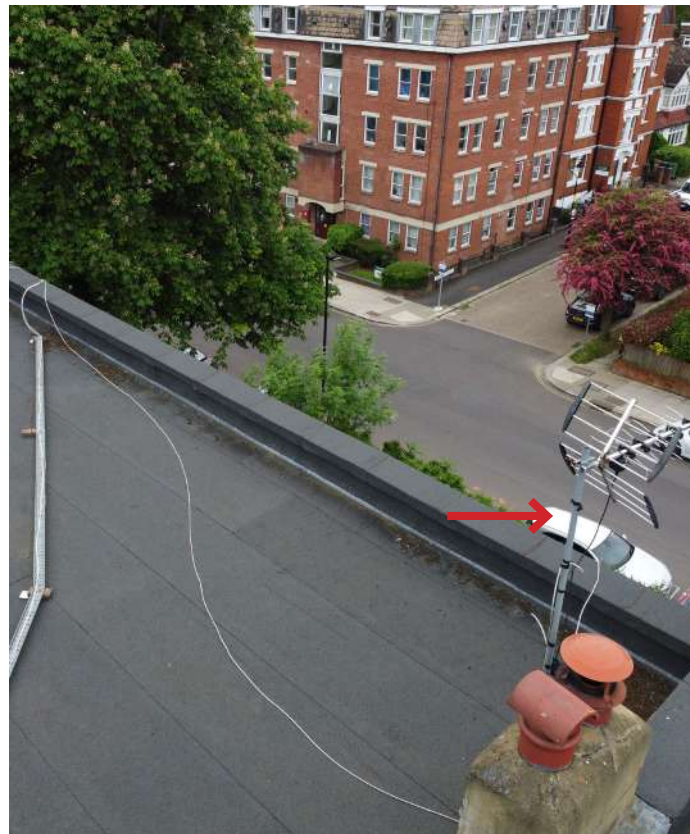
b. Cables, aerials and satellite dishes have built up on the roof and parapets creating an overall messy appearance.
