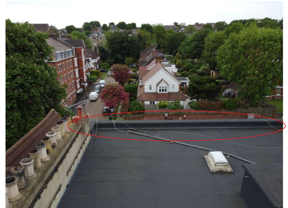
c. Low quality materials (felt) have been used on the roof and need to be replaced. The parapet height is very low and the waterproofing detail is not robust.
