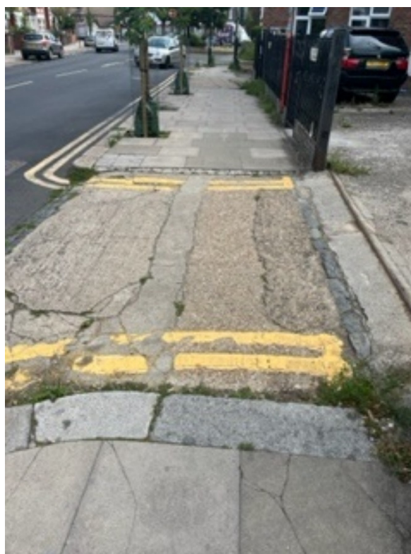
Photograph 4.5: Access road along the southern side of Lansdowne Road with no tactile paving and uneven dropped kerbs (looking south)
