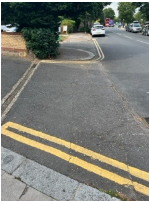
Photograph 4.6: Garwood Close access along the southern side of Lansdowne Road with no tactile paving and uneven dropped kerbs (looking north)
