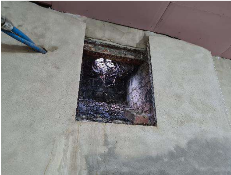
Figure 9: Vents into the basement from street level, which all appear well-sealed.
